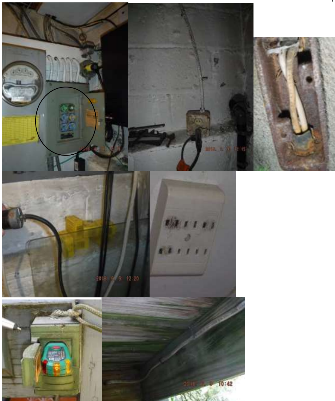
Figure 15 Examples of the old glass 6 fuse panel and older electrical. The home needs electrical upgrades throughout the home.
