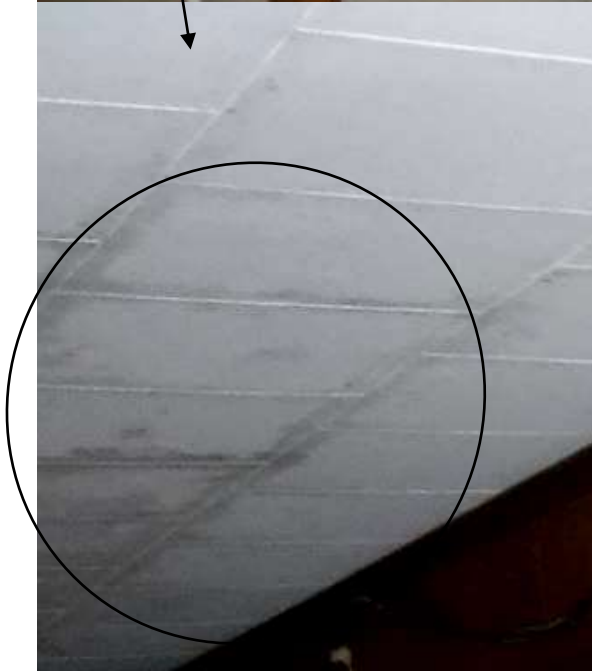
Figure 13 Finished basement (concealed structure) and mold-like spotting on ceiling tiles or surfaces. Follow-up with a mold or environmental contractor for that service and inspection; beyond the scope of a home inspection.
