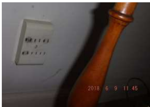
Figure 7 Example of multiplier on outlets and scorch marks; not recommended for fire safety.
