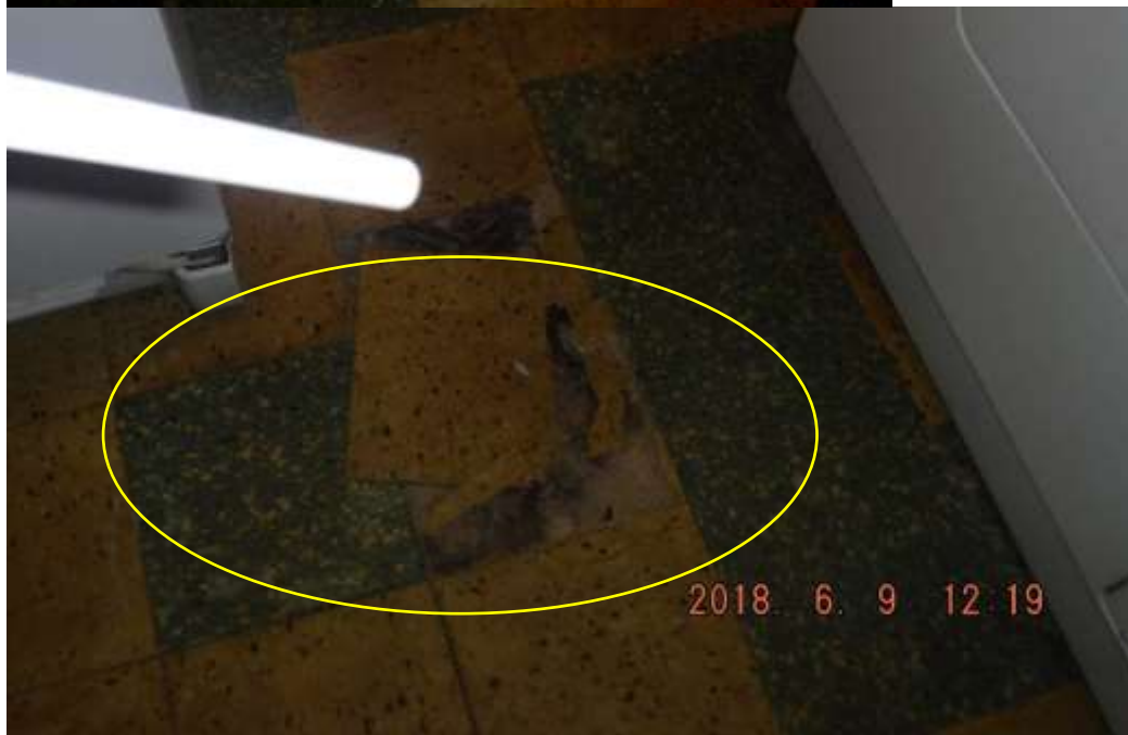
Figure 14 Example of asbestos-like floor tiles; water damaged/broken. Follow-up with an asbestos or environmental contractor.
