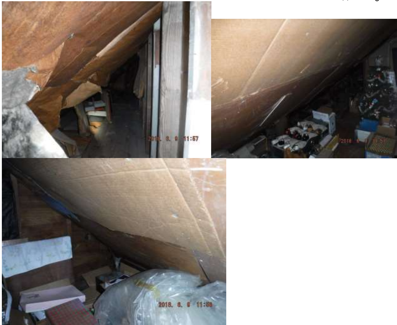
Figure 3 Insulation & cardboard against the rafters; improper installation. Insulation should be on the living spaces or knee walls to avoid condensation build-up, heat and moisture damage.
