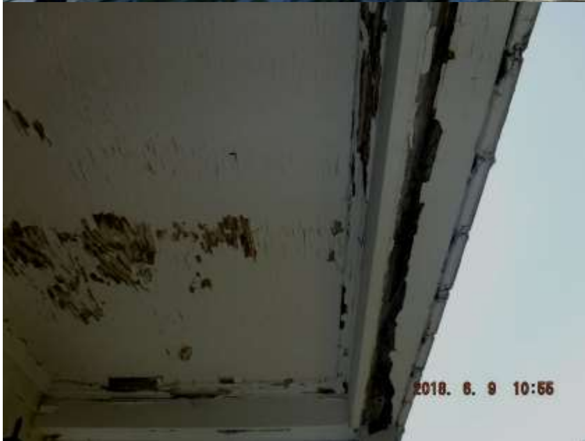
Figure 5 Examples of siding/exterior rot and peeled paint; poorly maintained exterior & systems.
