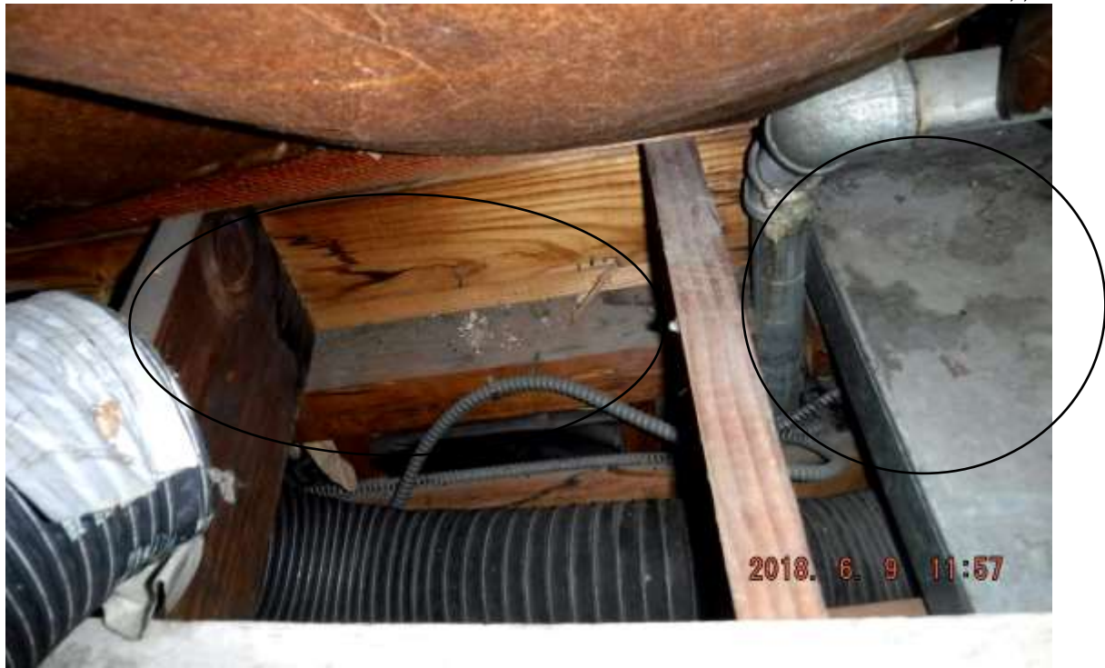
Figure 2 Example of water stains/active leaking in attic.
