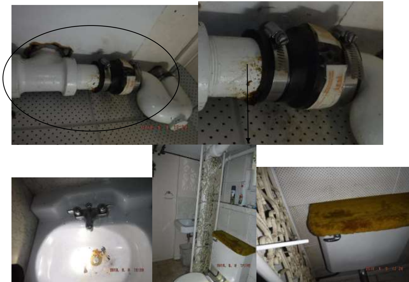
Figure 6 Basement 1/2 bathroom was not functional; do not use. Have a bathroom contractor evaluate and advise on complete renovations, plumbing, electrical, etc.
