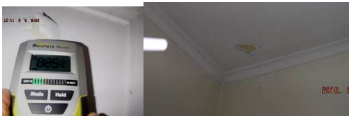
Figure 9 Example of flaked paint, water stains and active moisture/leaking; see roofing section comments.
