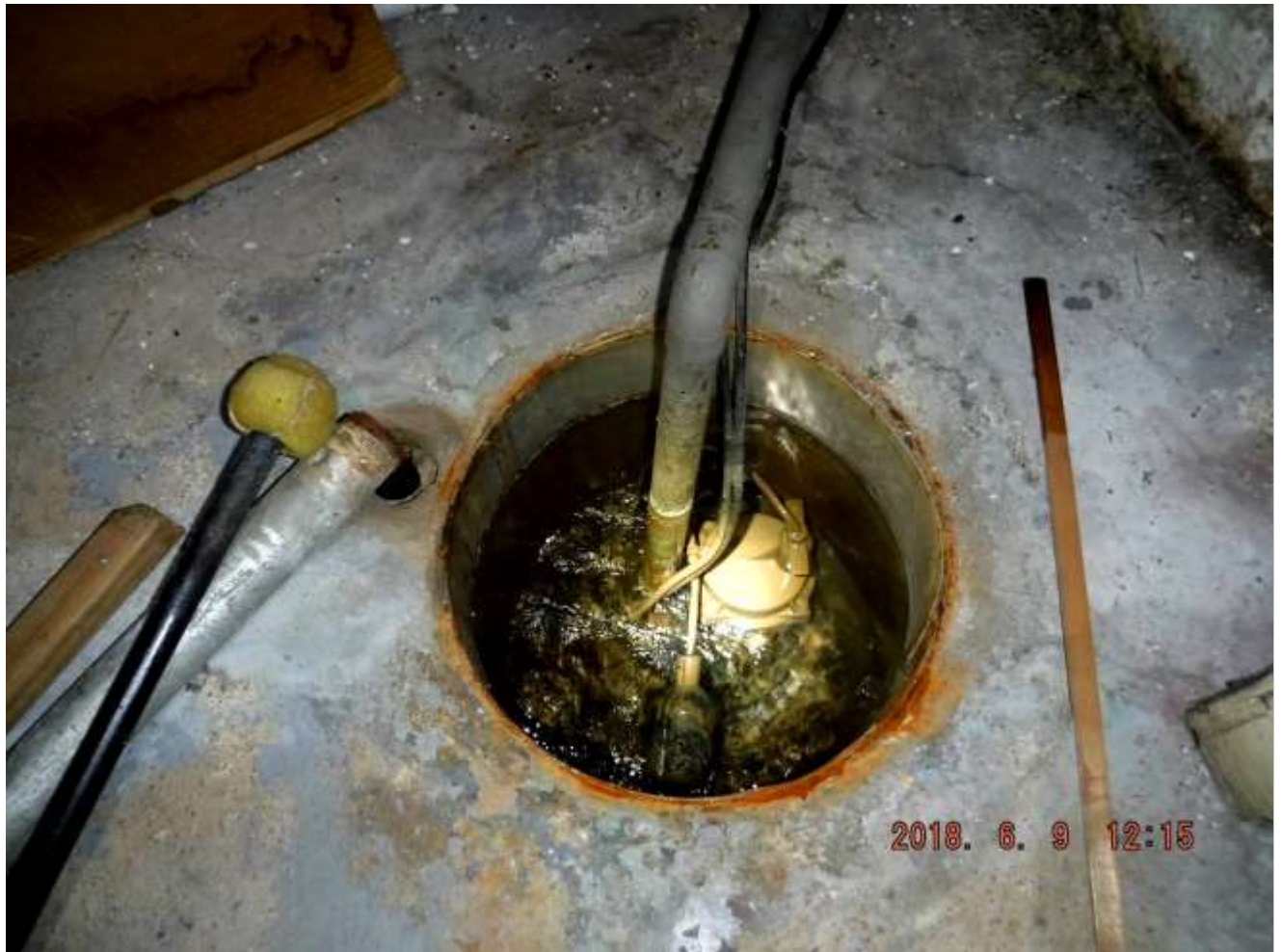
Figure 12 Sump was nearly filled, no check valves, no cover, no dedicated outlet/GFCI, etc.
