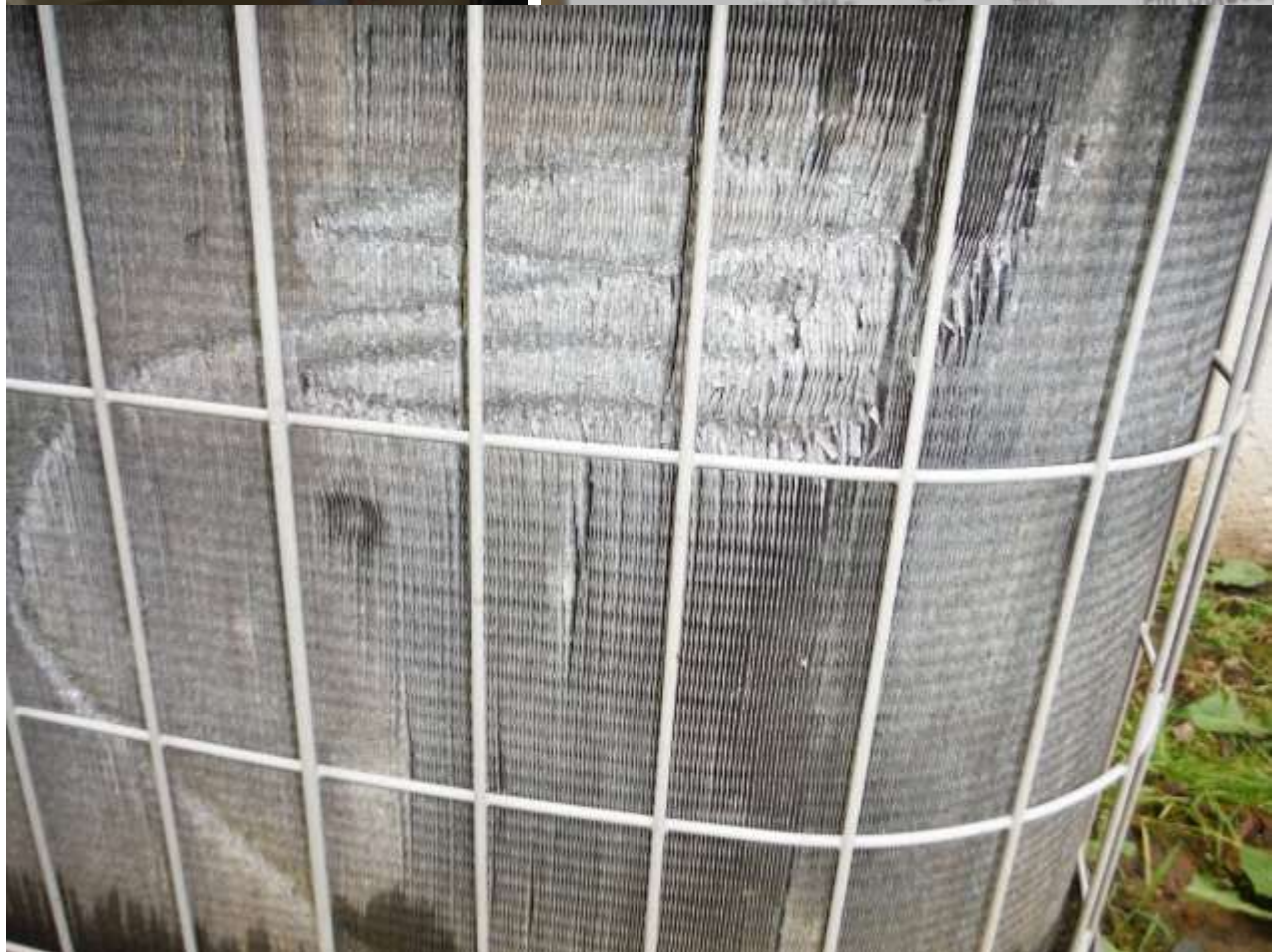
Figure 8 York condenser SN# WFKM010373 (K=2001)*- past expected life/damaged fins & not cooling properly.
