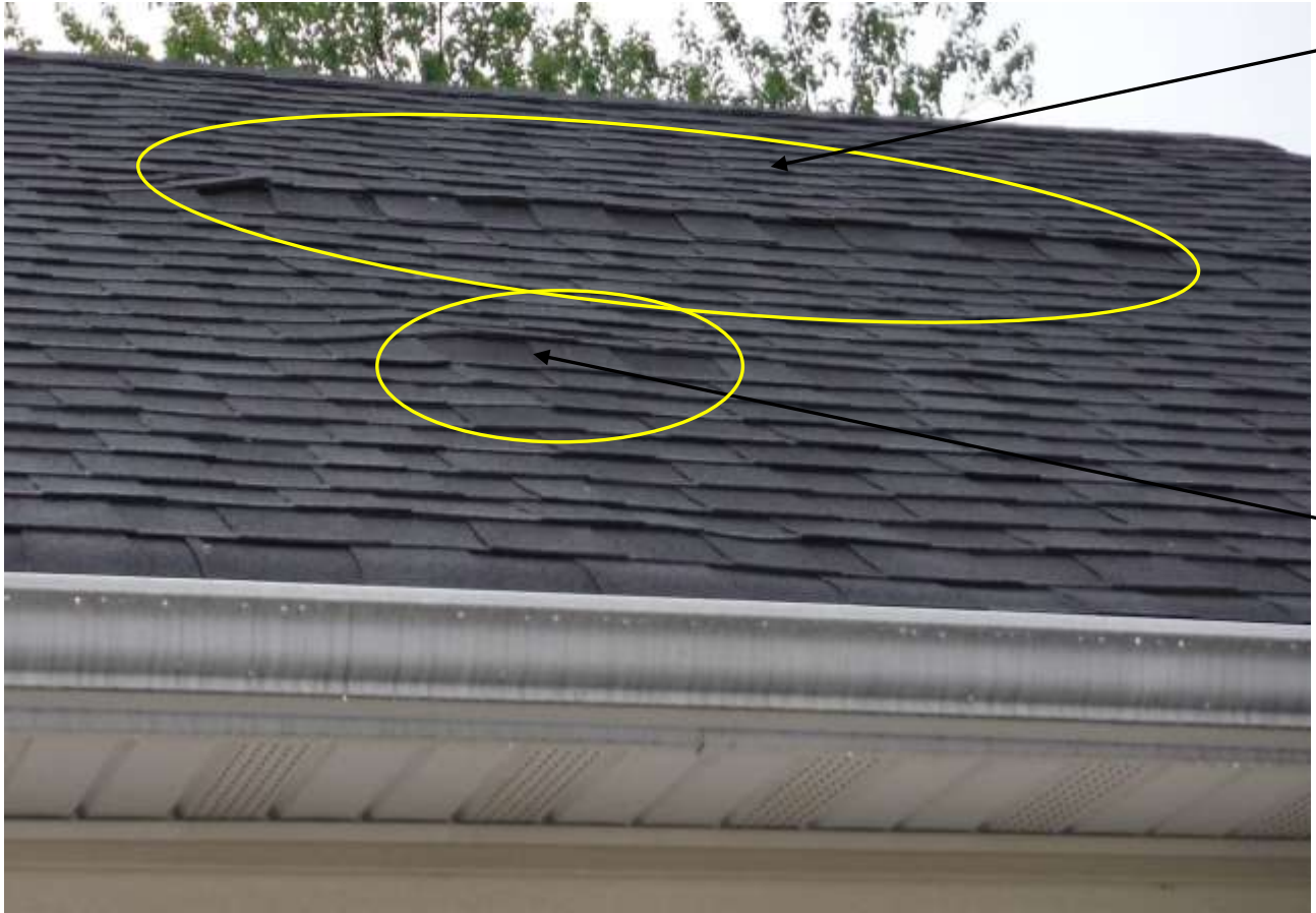
Figure 2 Have a qualified roofer evaluate roof and make repairs where needed; lifted shingles/humps on roof. See attic section comments.
