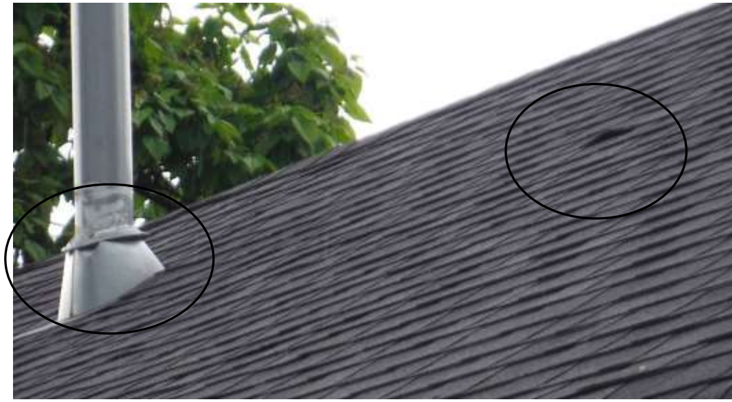
Figure 3 Chimney dented/crimped, white condensate visible in attic; drafting concerns. Chimney was not installed properly; safety hazard/dangerous. Water entry points at gaps on chimney.
