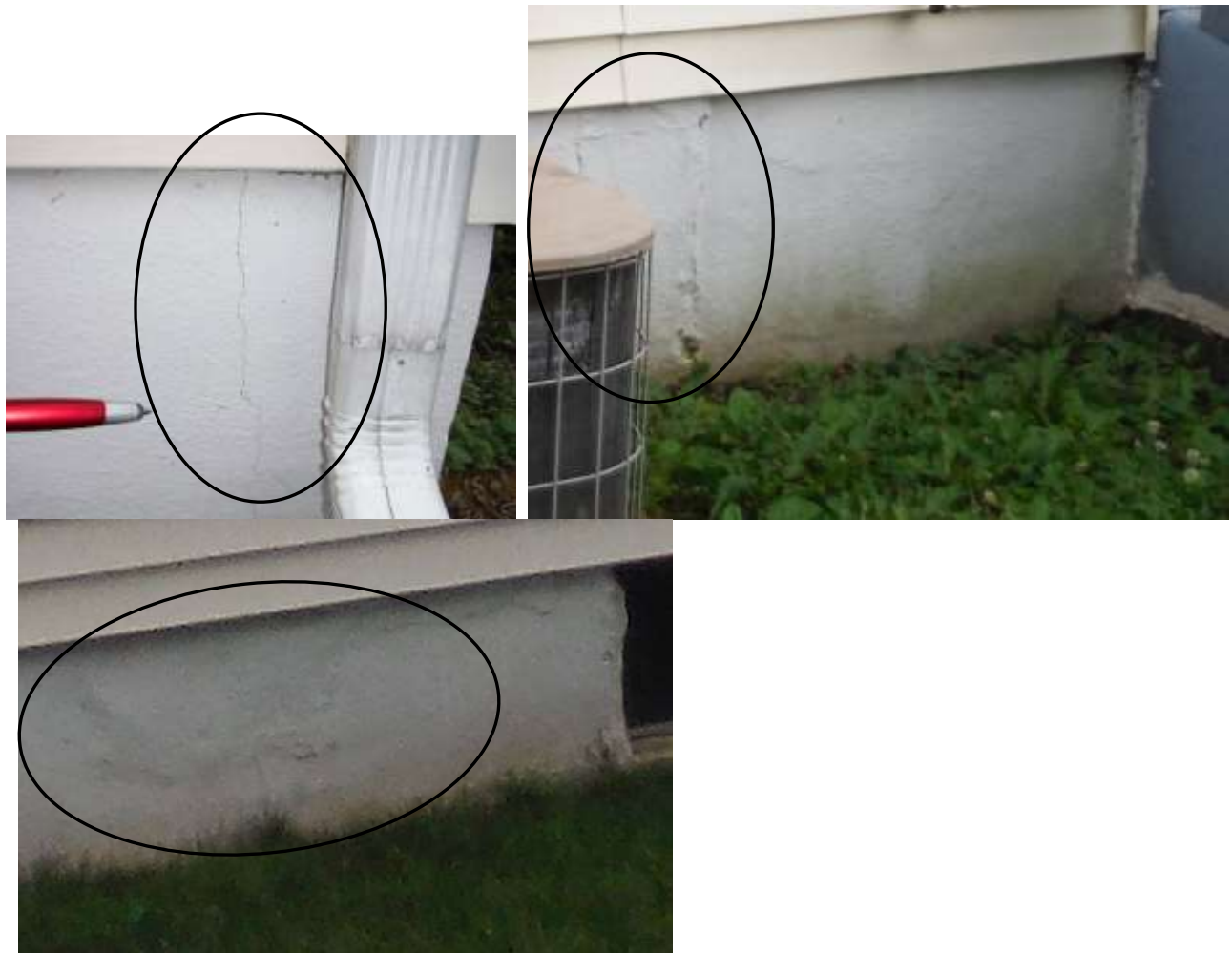
Figure 5 Examples of foundation cracks & patched cement on home as viewed from exterior. Have a foundation repair contractor or structural mason evaluate/repair all cracks/damage where needed. Inspect basement & crawl spaces when made accessible; see basement & crawl space section comments.
