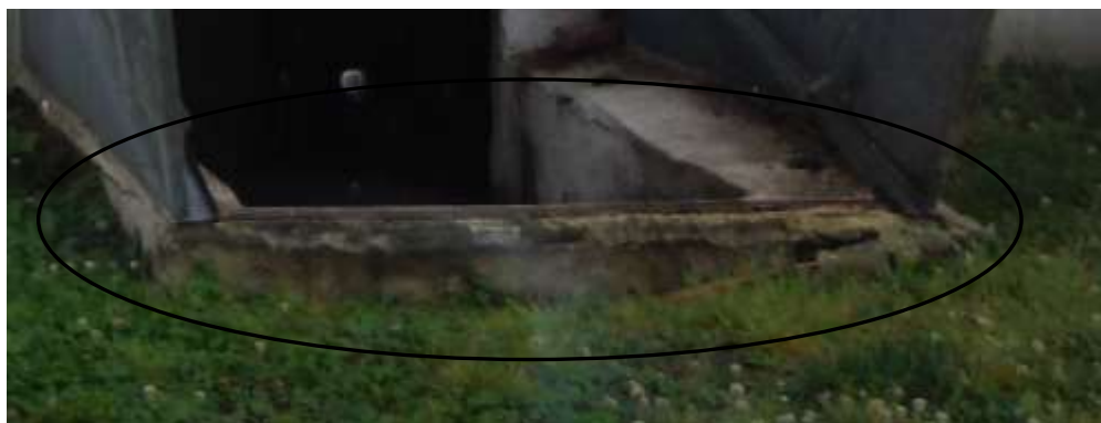
Figure 1 Water damaged concrete on the Bilco curbing and basement walkout.
