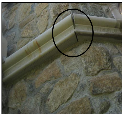
Figure 18 Gaps around rear patio cement
