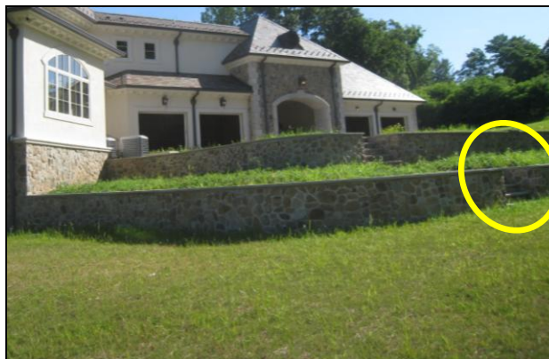
Figure 30 No railings, missing walk connecting walls
