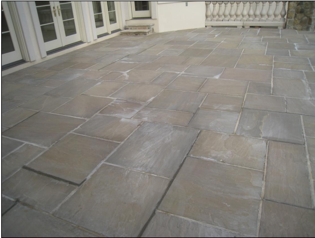
Figure 34 Many mortar repairs being made on patio. Some areas or joints raised.
