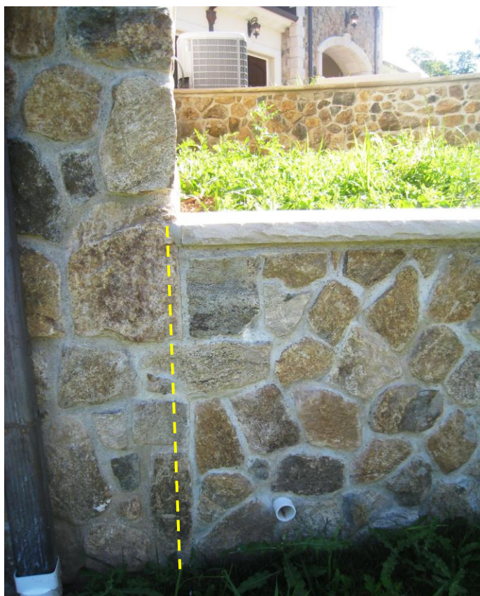
Figure 9 Vertical cracks at retaining wall/siding juncture
