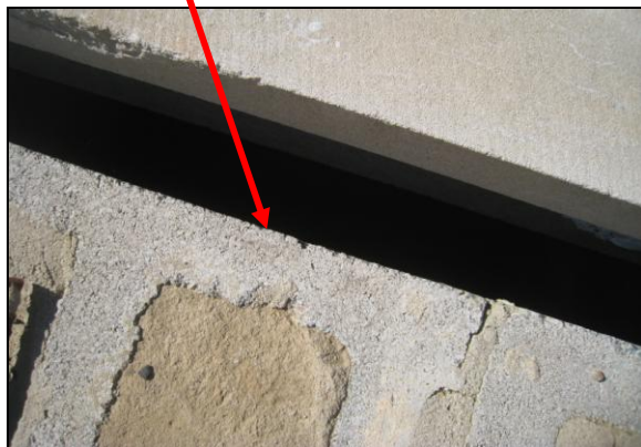
Figure 29 Wide gap, stagnant water inside below lower steps; drainage & safety concerns.
