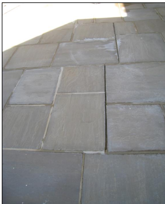
Figure 5 Gaps in patio off living room.
