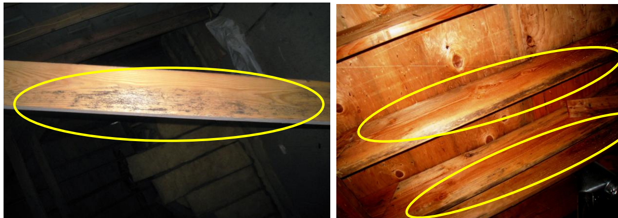
Figure 26 Examples of Possible mold; further evaluate and mitigate as per contractor & testing.
