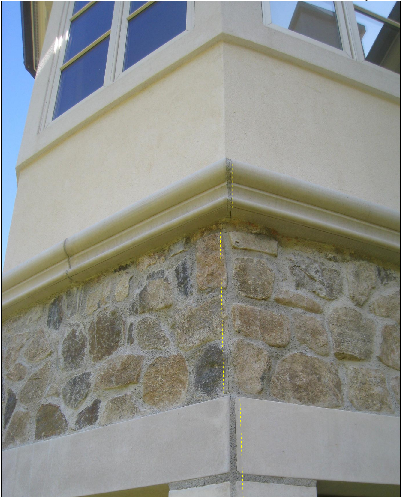
Figure 22 Examples of vertical cracks all around kitchen outcrop
