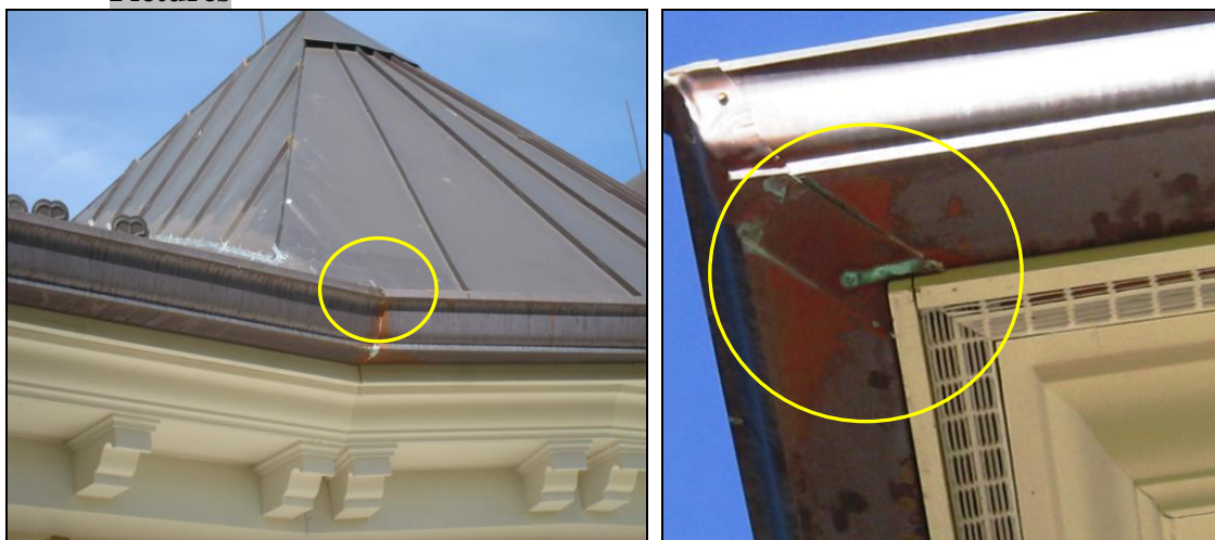
Figure 14 A & B Leaking at junctures
