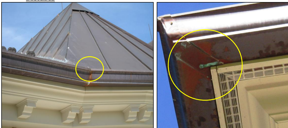
Figure 41 A &amp; B Leaking at junctures
