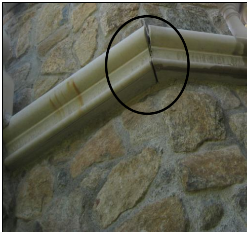
Figure 45 Gaps around rear patio cement
