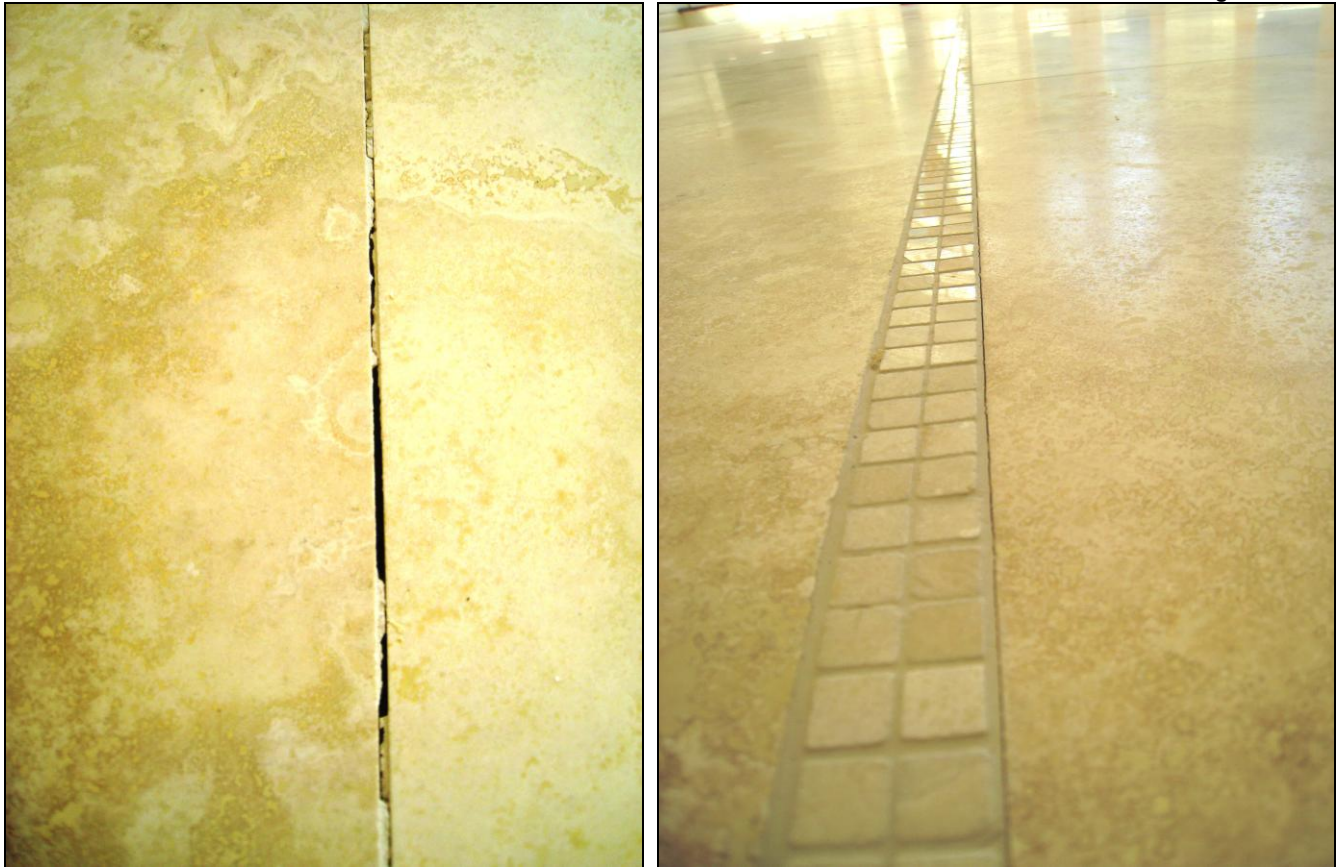
Figure 24 Numerous cracks on tiled flooring in living room; have evaluated and corrected.
