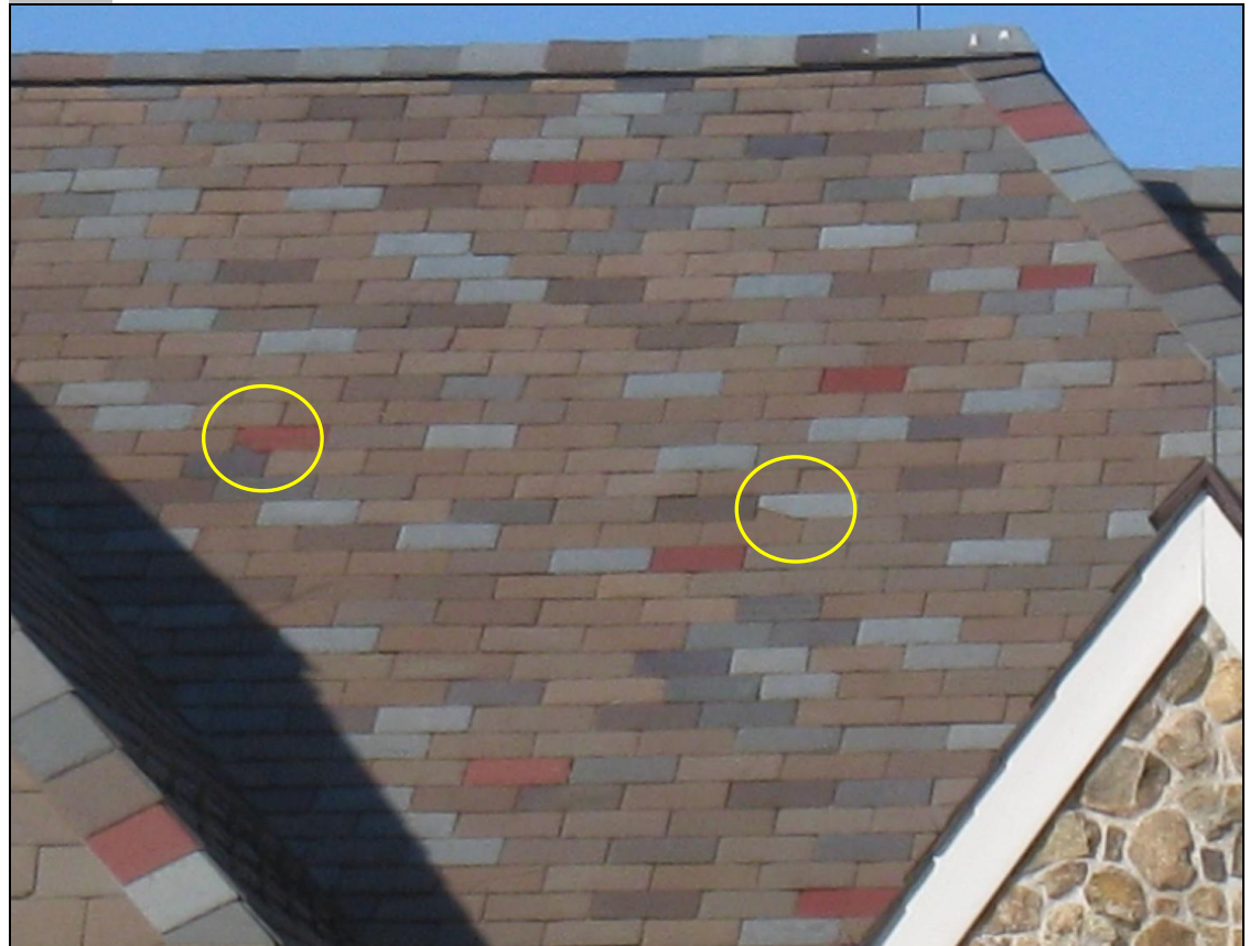
Figure 37 Examples of broken shingles
