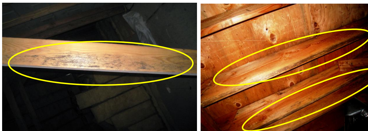
Figure 53 Examples of Possible mold; further evaluate and mitigate as per contractor & testing.
