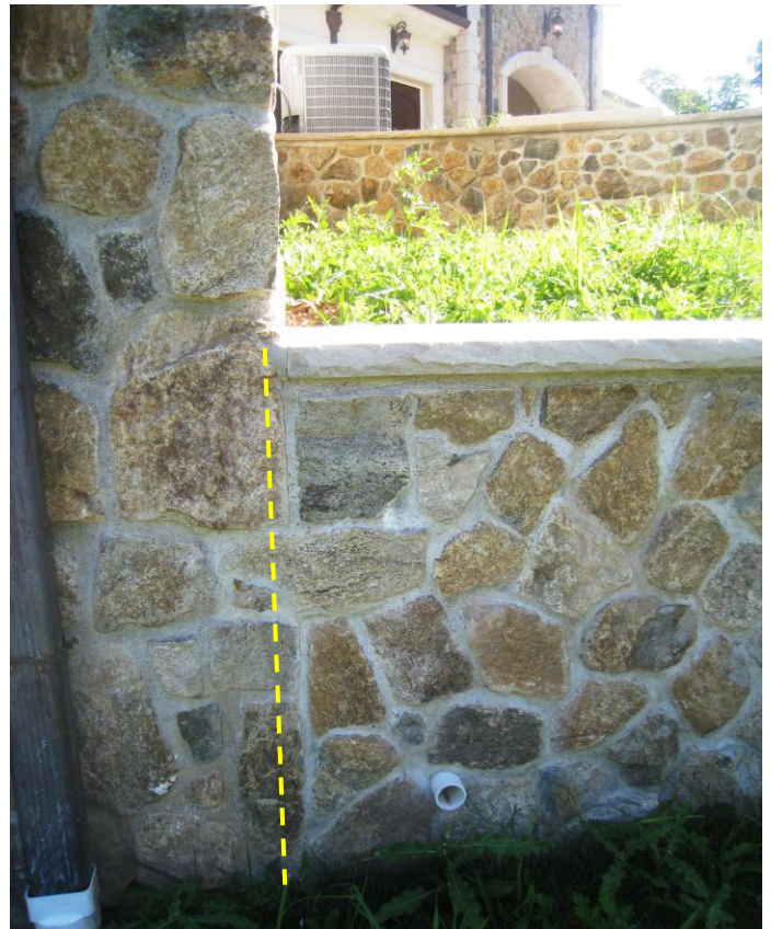
Figure 36 Vertical cracks at retaining wall/siding juncture
