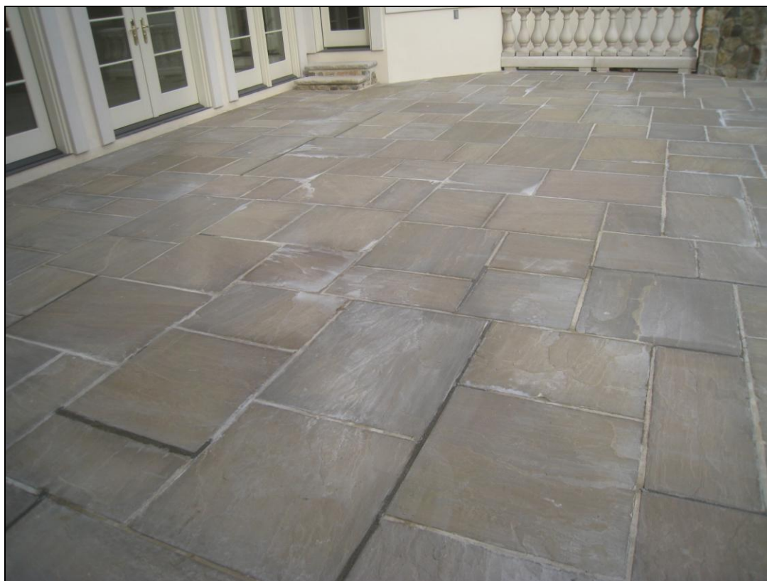
Figure 7 Many mortar repairs being made on patio. Some areas or joints raised.
