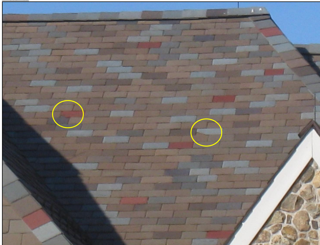
Figure 10 Examples of broken shingles
