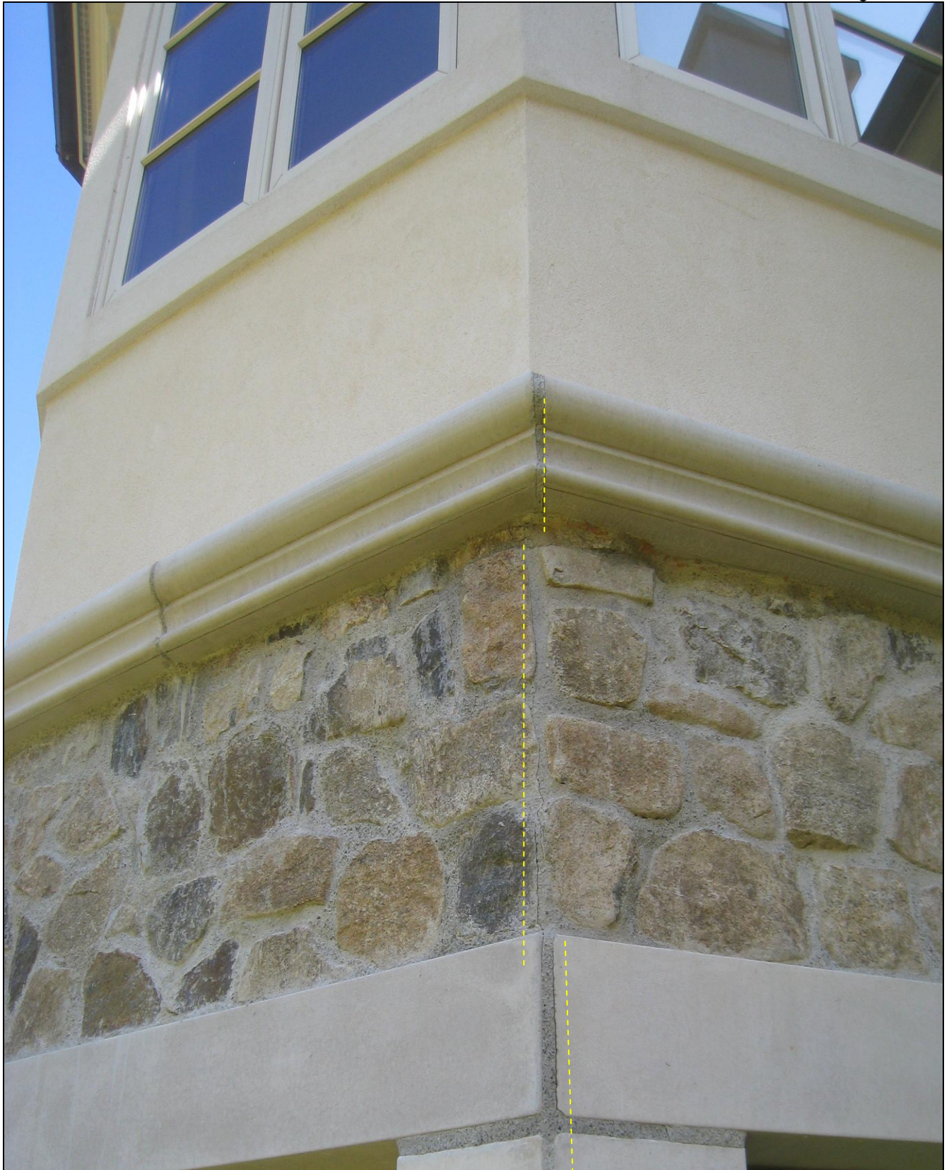
Figure 49 Examples of vertical cracks all around kitchen outcrop
