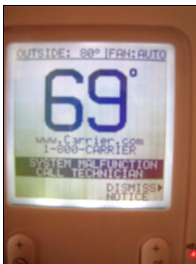
Figure 54 # Units gave this message when heat or HVAC tested.
