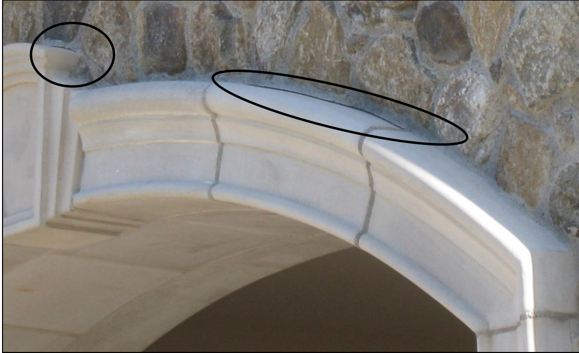
Figure 44 Gaps, mortar or caulking needed.
