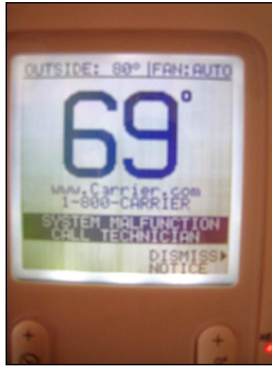
Figure 27 # Units gave this message when heat or HVAC tested.
