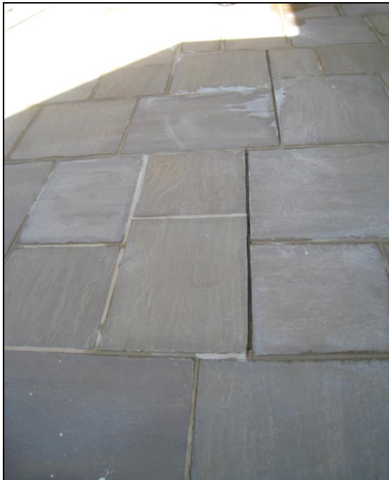
Figure 32 Gaps in patio off living room.
