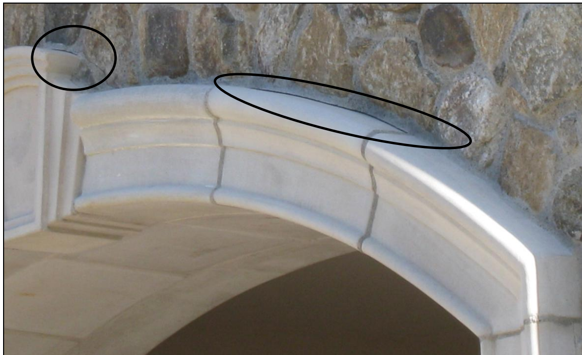
Figure 17 Gaps, mortar or caulking needed.
