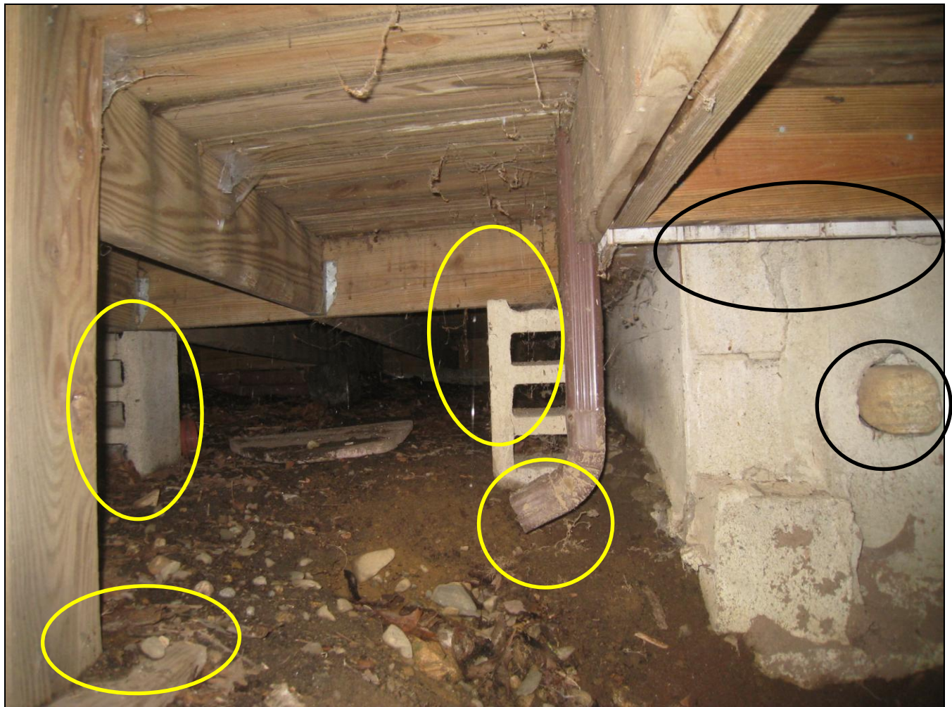
Figure 13 Deck improper construction; structural safety concern. Rain leader discharging near foundation; water infiltration and soil erosion. There is a rock stuffed into a hole on foundation; unconventional repair.
