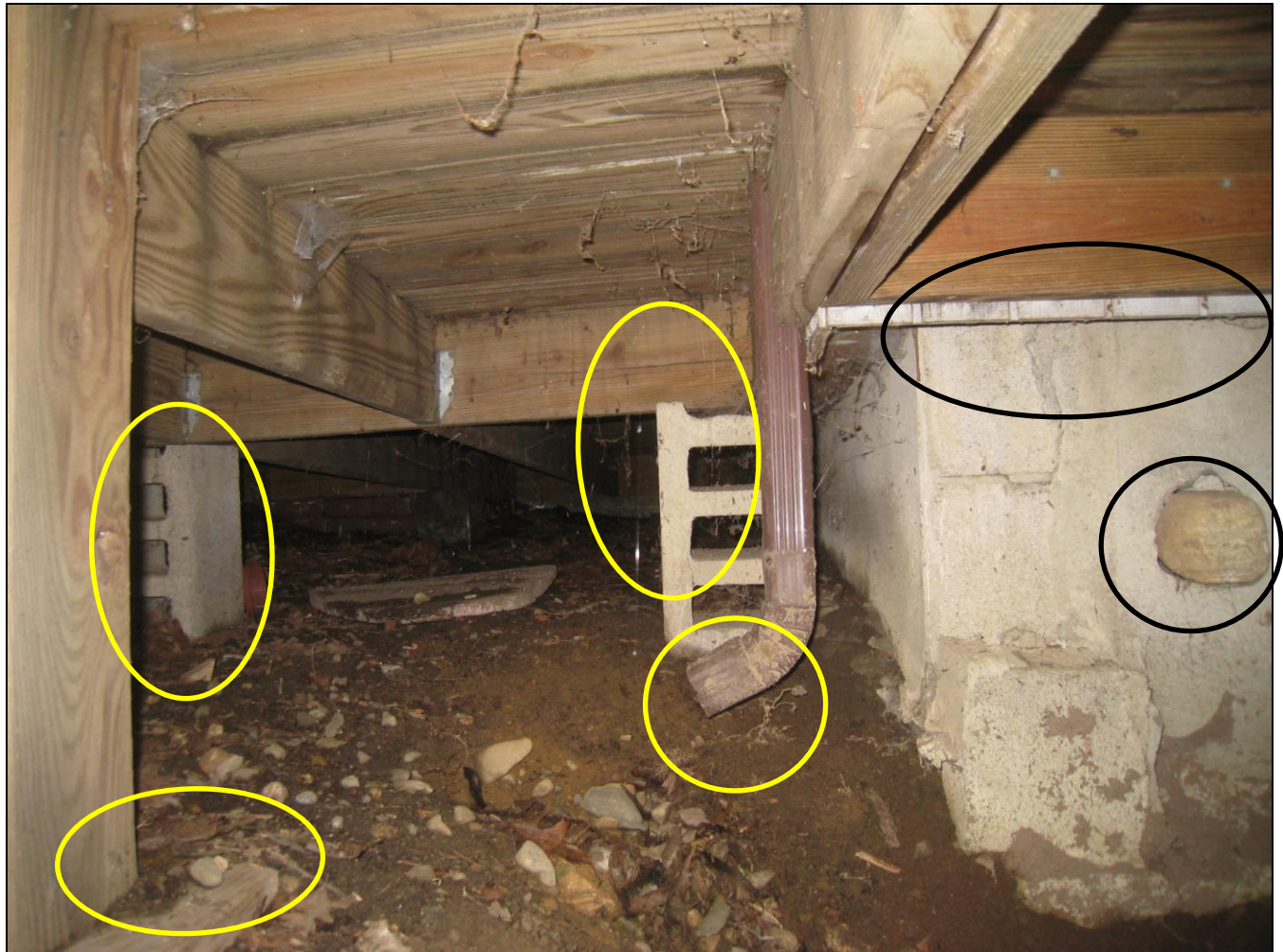
Figure 4 Deck improper construction; structural safety concern. Rain leader discharging near foundation; water infiltration and soil erosion. There is a rock stuffed into a hole on foundation; unconventional repair.
