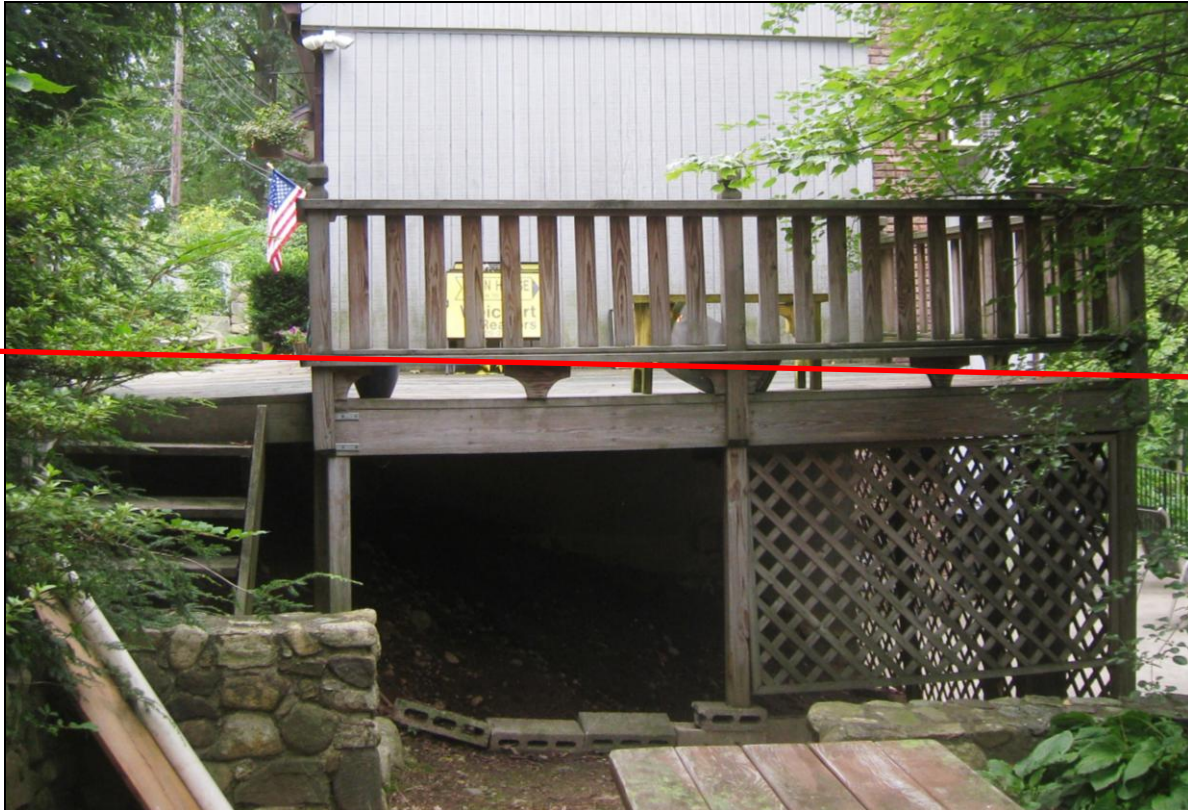
Figure 10 Deck sloped, not properly attached to house, no flashings, no footings for vertical columns & steps, railings too low; unsafe structure.
