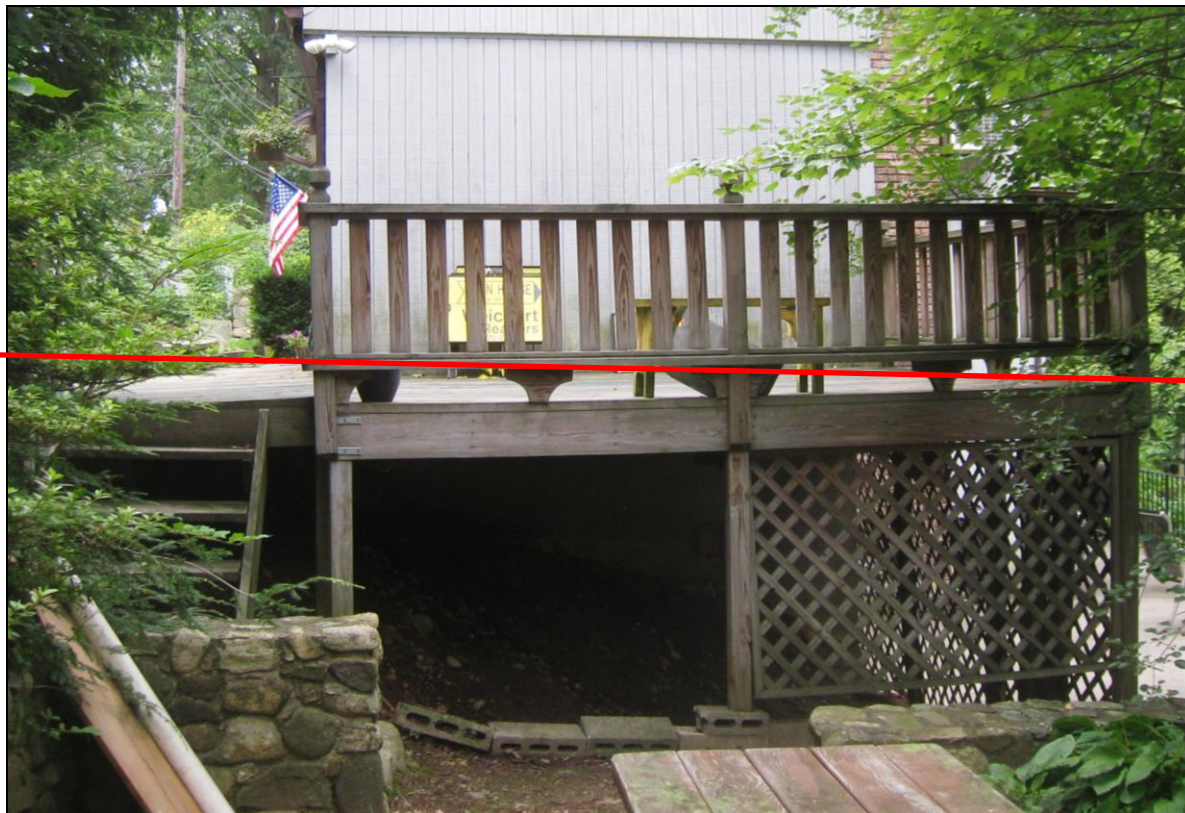
Figure 1 Deck sloped, not properly attached to house, no flashings, no footings for vertical columns & steps, railings too low; unsafe structure.
