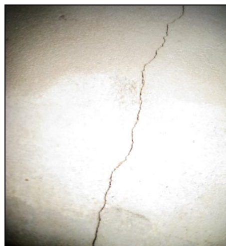
Figure 12 Examples of foundation cracks; evaluate.
