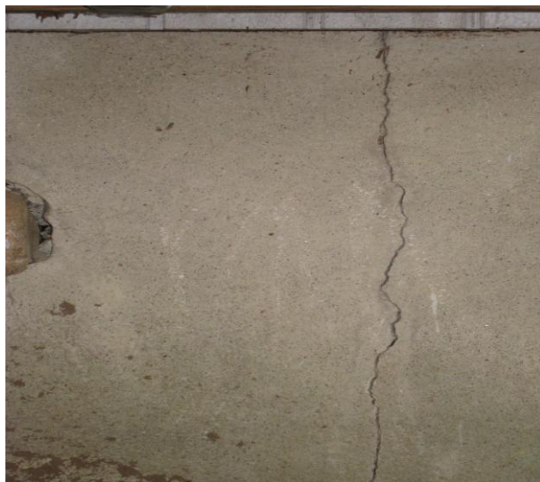
Figure 14 Foundation cracks visible under decking; have evaluated with structure.
