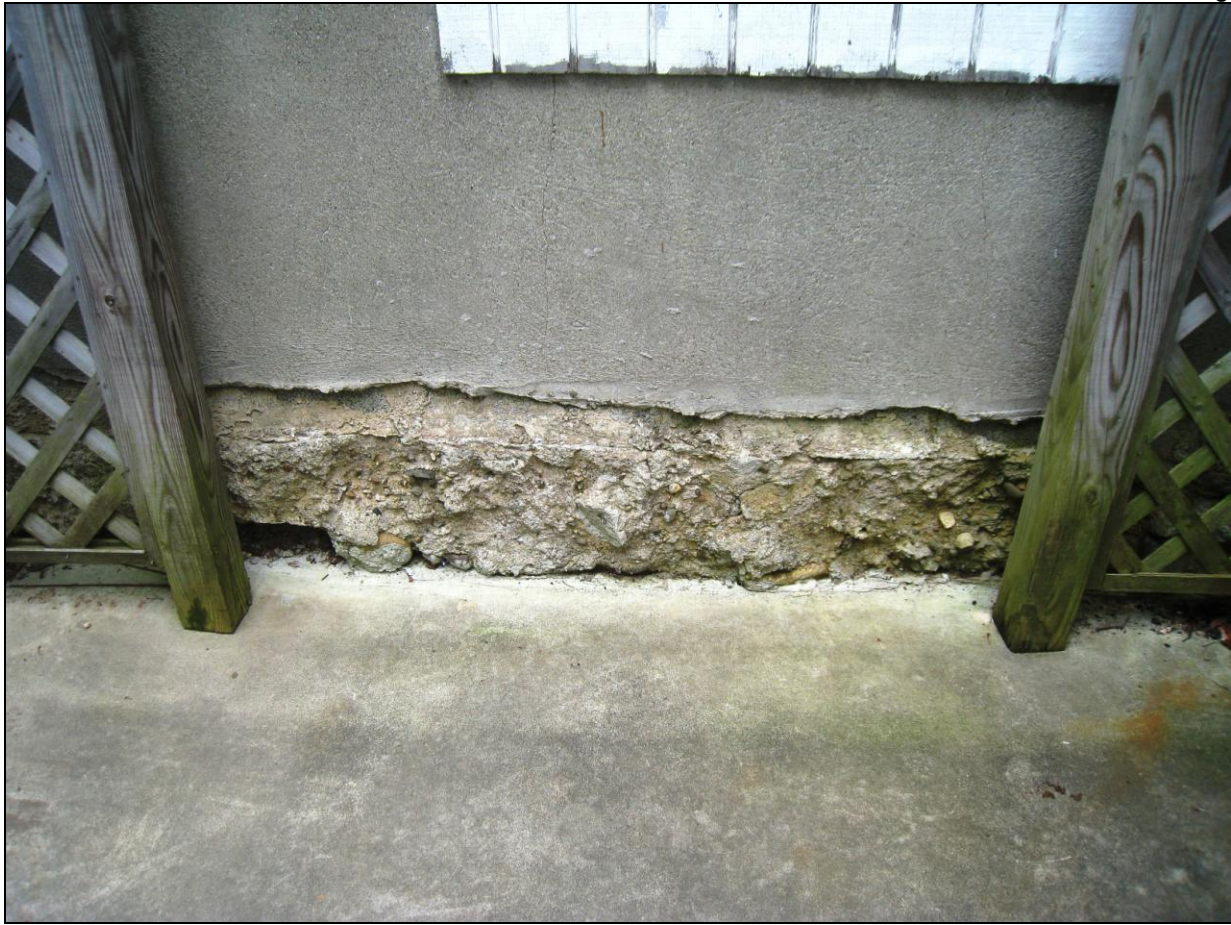
Figure 16 Exposed footers on crawl ; view from concrete patio in rear. Have structure evaluated.
