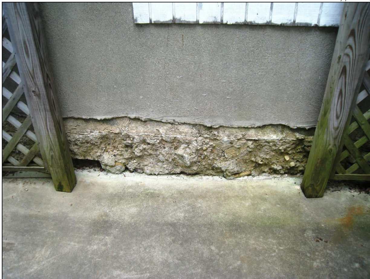
Figure 7 Exposed footers on crawl ; view from concrete patio in rear. Have structure evaluated.
