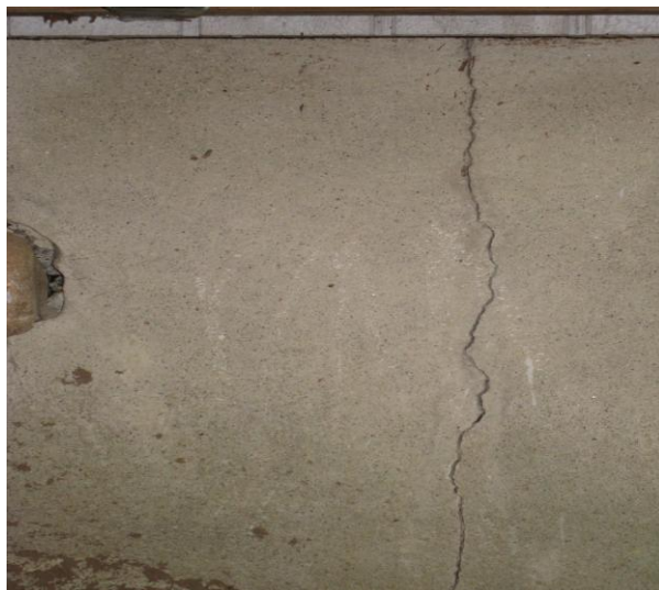
Figure 5 Foundation cracks visible under decking; have evaluated with structure.
