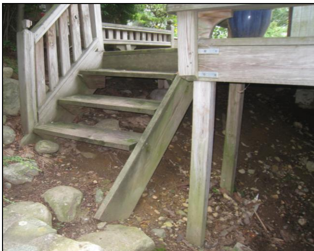
Figure 11 Deck steps improperly supported/constructed.
