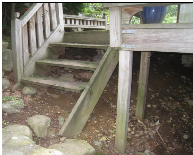
Figure 2 Deck steps improperly supported/constructed.
