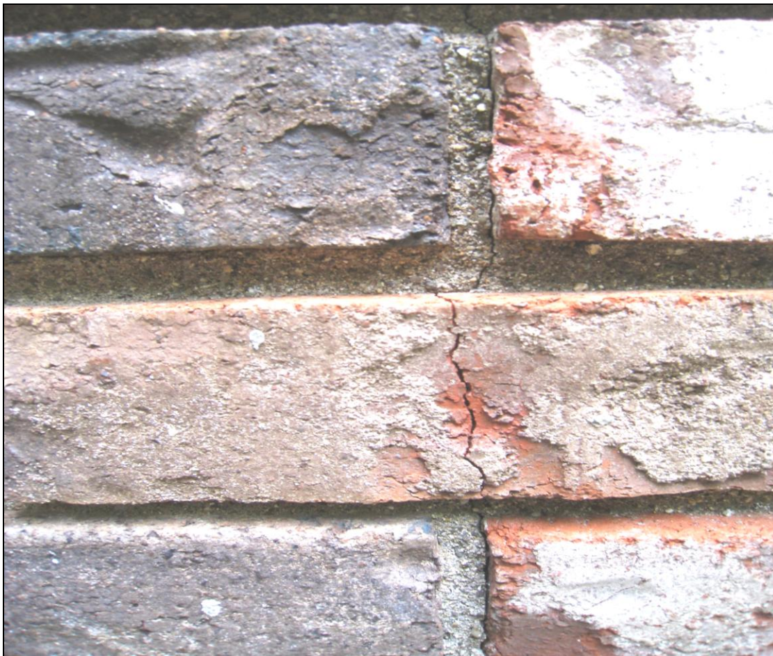
Figure 17 Example of cracks through brick and mortar on rear chimney; have chimney contractor evaluate
