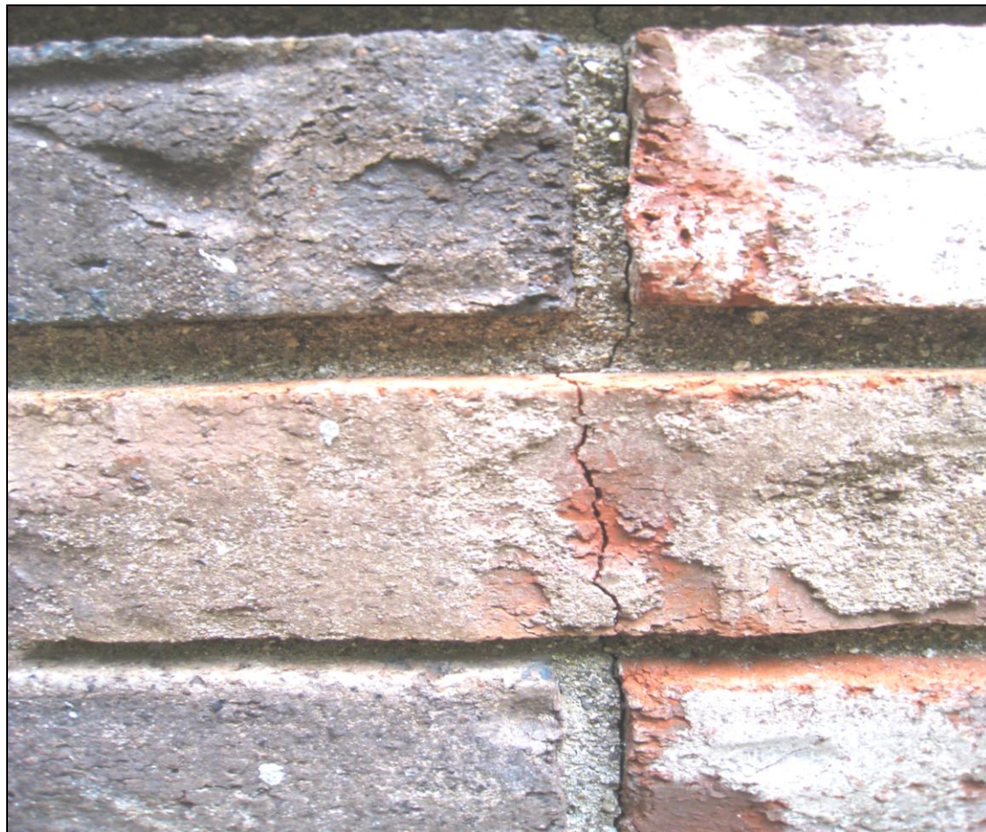
Figure 8 Example of cracks through brick and mortar on rear chimney; have chimney contractor evaluate
