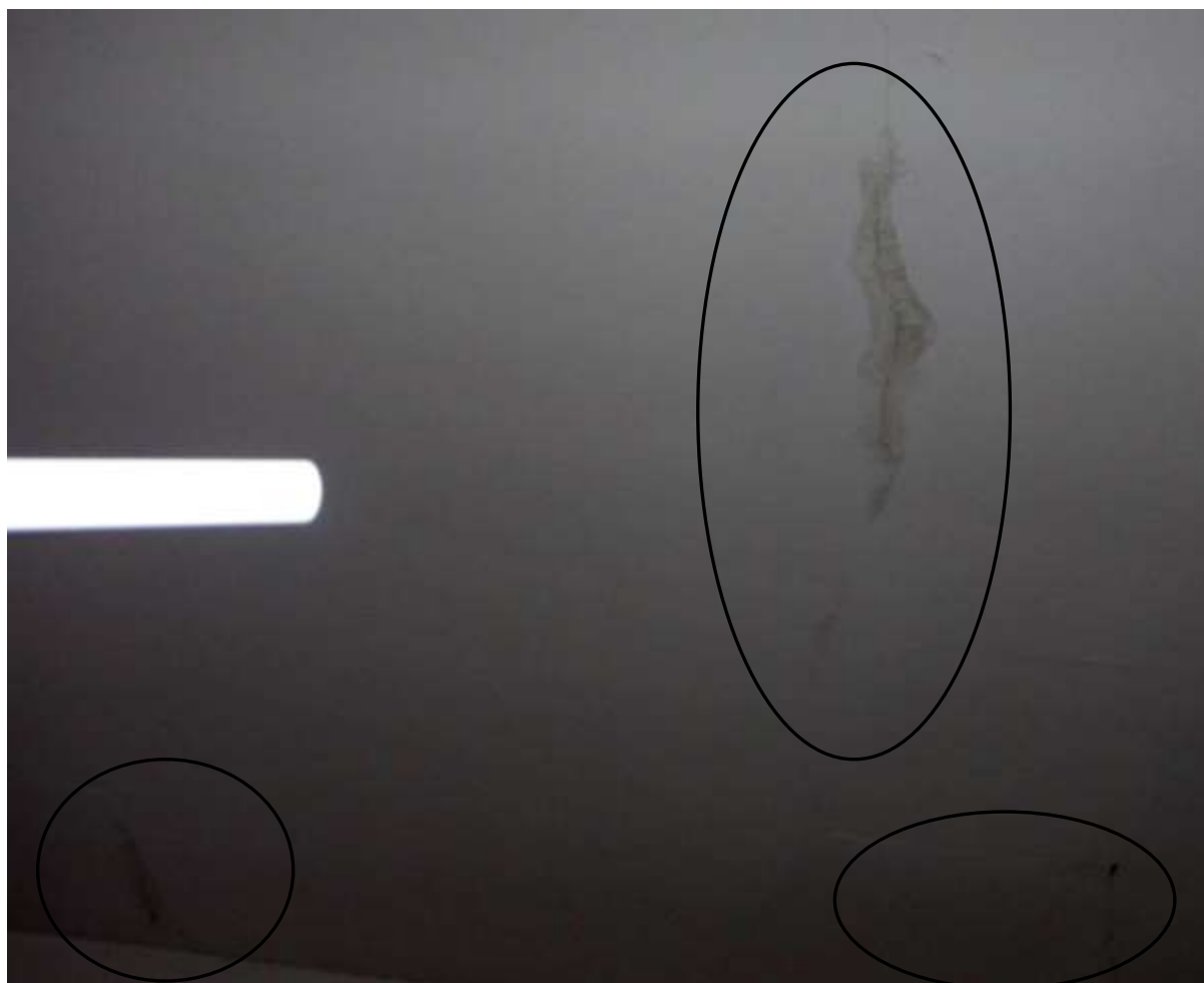
Example of active leaks in interior of home (ceilings, closets, etc.). Recommend a building contractor & roofer evaluate exterior and advise on all repairs and sources of water. Exterior poorly maintained.
