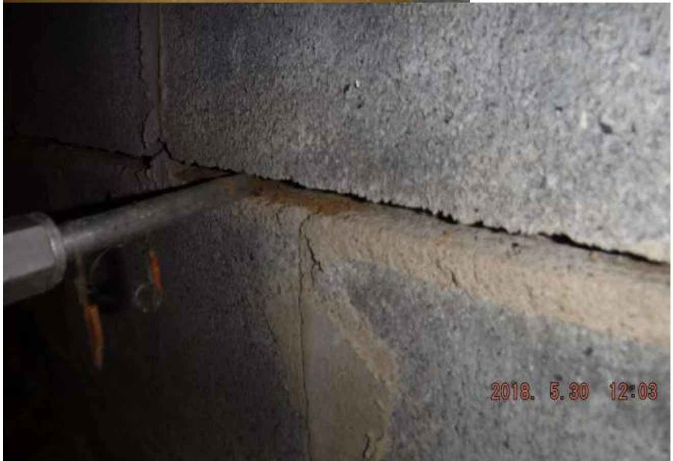
Figure 16 Example of areas with approximately 1/2" opening are bowed wall(s).
