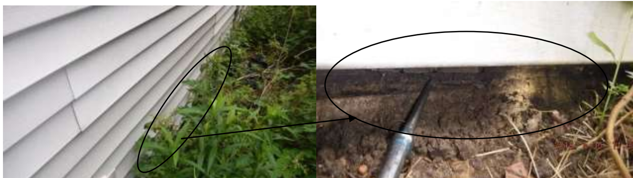
Figure 10 Example of moisture and termite damage on slab construction; limited view due to high weeds or overgrowth. See structural comments in crawl space and pg.2. main concerns. There was extensive termite damage on sills in crawl space; limited access due to low height in crawl.
