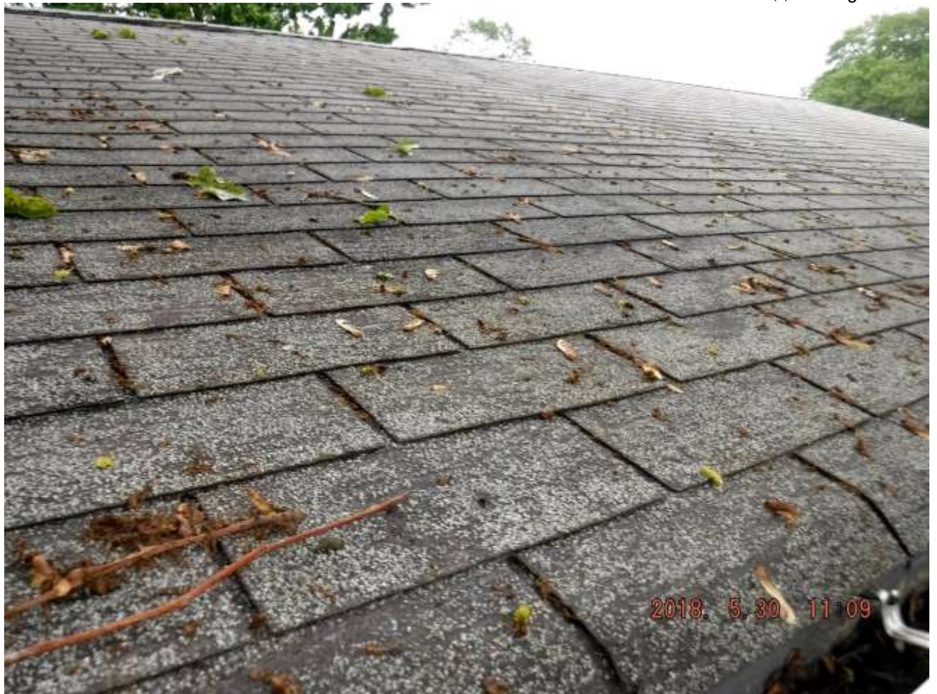
Figure 3 Much of the granules or aggregate was gone and backing visible or exposed.
