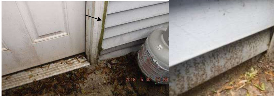
Figure 9 Example of siding in soil and buckled.
