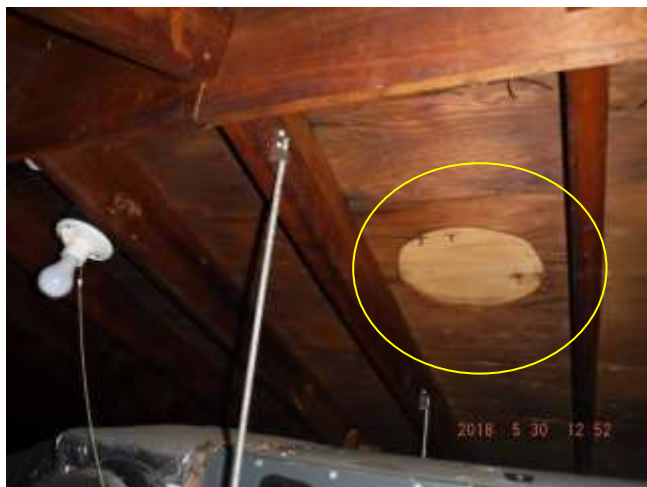
Figure 6 Example of closed roof fan(s); poor ventilation in attic.
