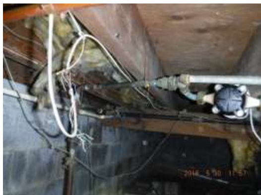
Figure 18 Partial view of water meter & gate valve shutoff. Gate valves tend to stick, leak and difficult to close to operate in an emergency. Recommend upgrading to single handle ball valves on main and in home.
