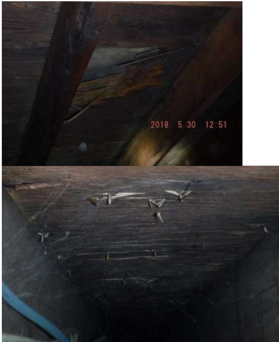
Figure 5 Example of sheathing splits/heat damage/brittle; poor ventilation.
