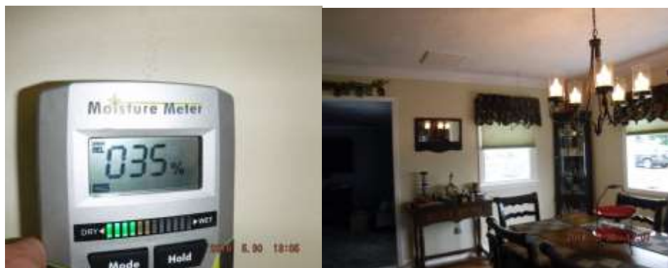
Figure 12 Moisture around windows when spot-checked; further evaluate by exterior/siding contractor.
