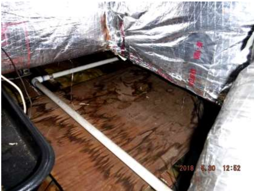
Figure 20 Example of condensate or water stains around the air handler in attic; recommend an HVAC contractor evaluate cooling system/service and advise before closing. Cooling not tested to avoid leaking or condensate damage should unit not function properly and potentially cause damage to interior rooms.
