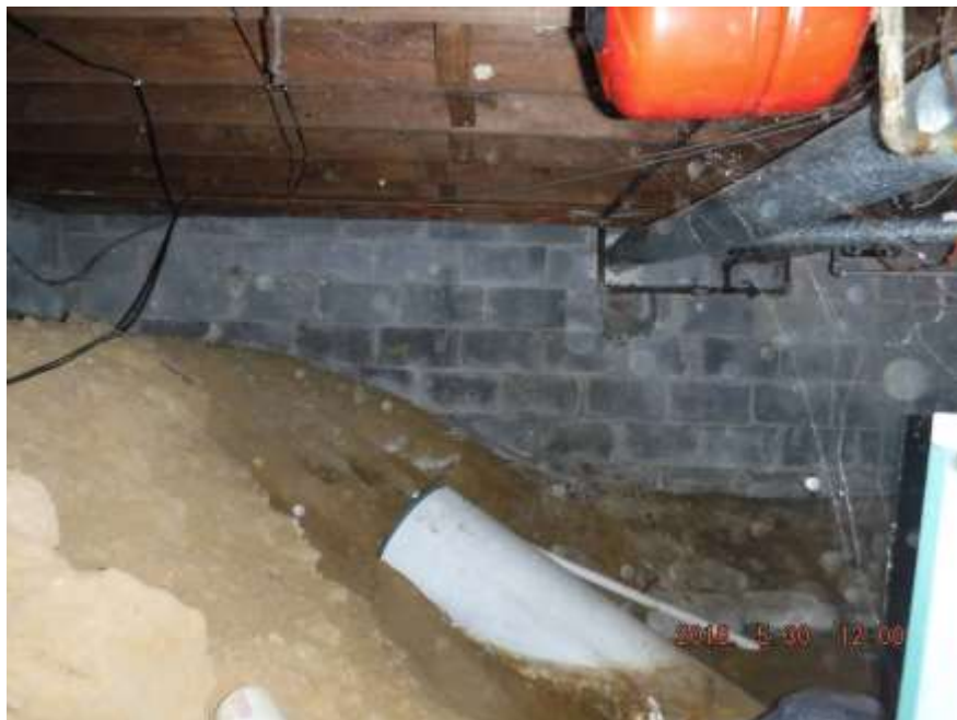
Figure 15 Example of depended dirt floor, foundation cracks, old water heater in dirt, wet dirt/seepage, etc.
