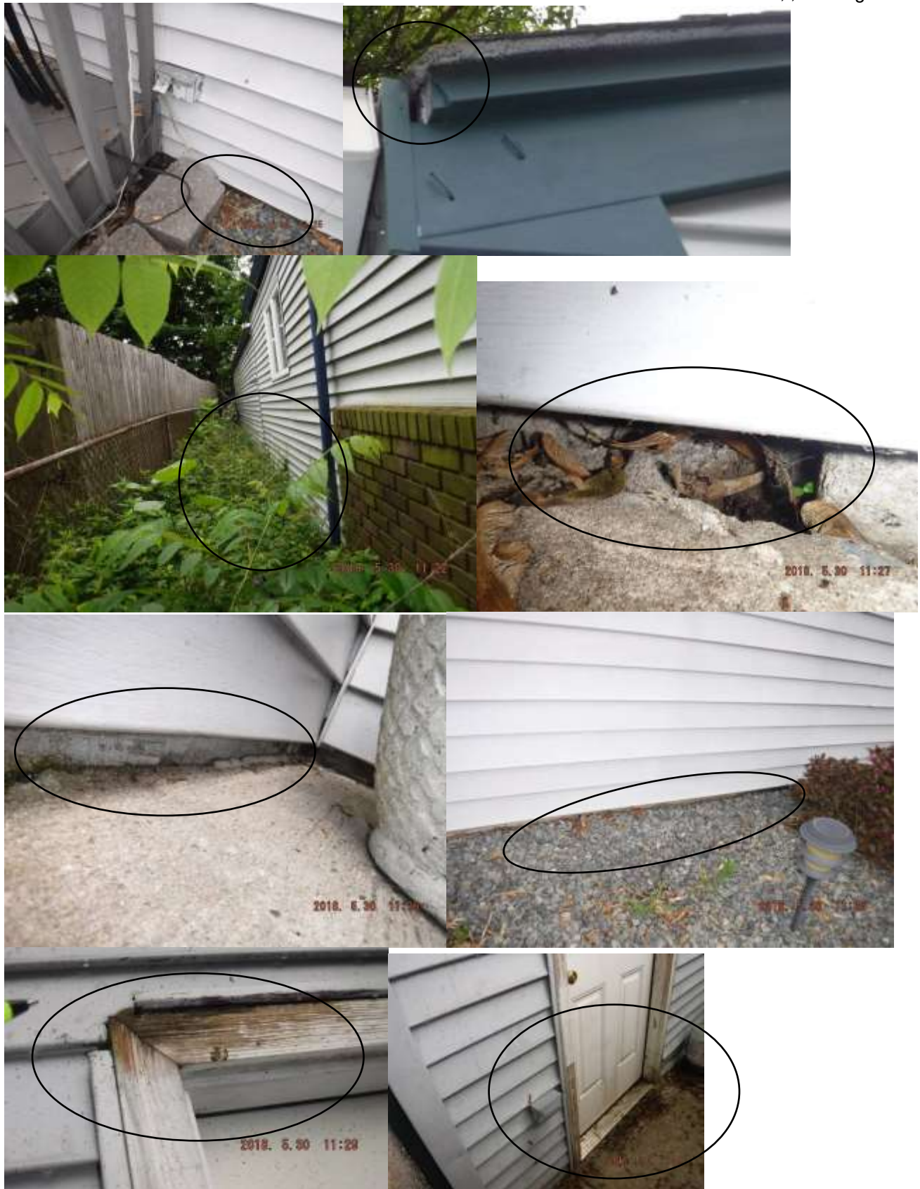
Figure 8 Examples of exterior siding: improper clearance, buckled siding, loose, gaps, improper trim/J-molding cuts, flashings missing or inadequate, cracks/gaps on slab foundation, etc.
