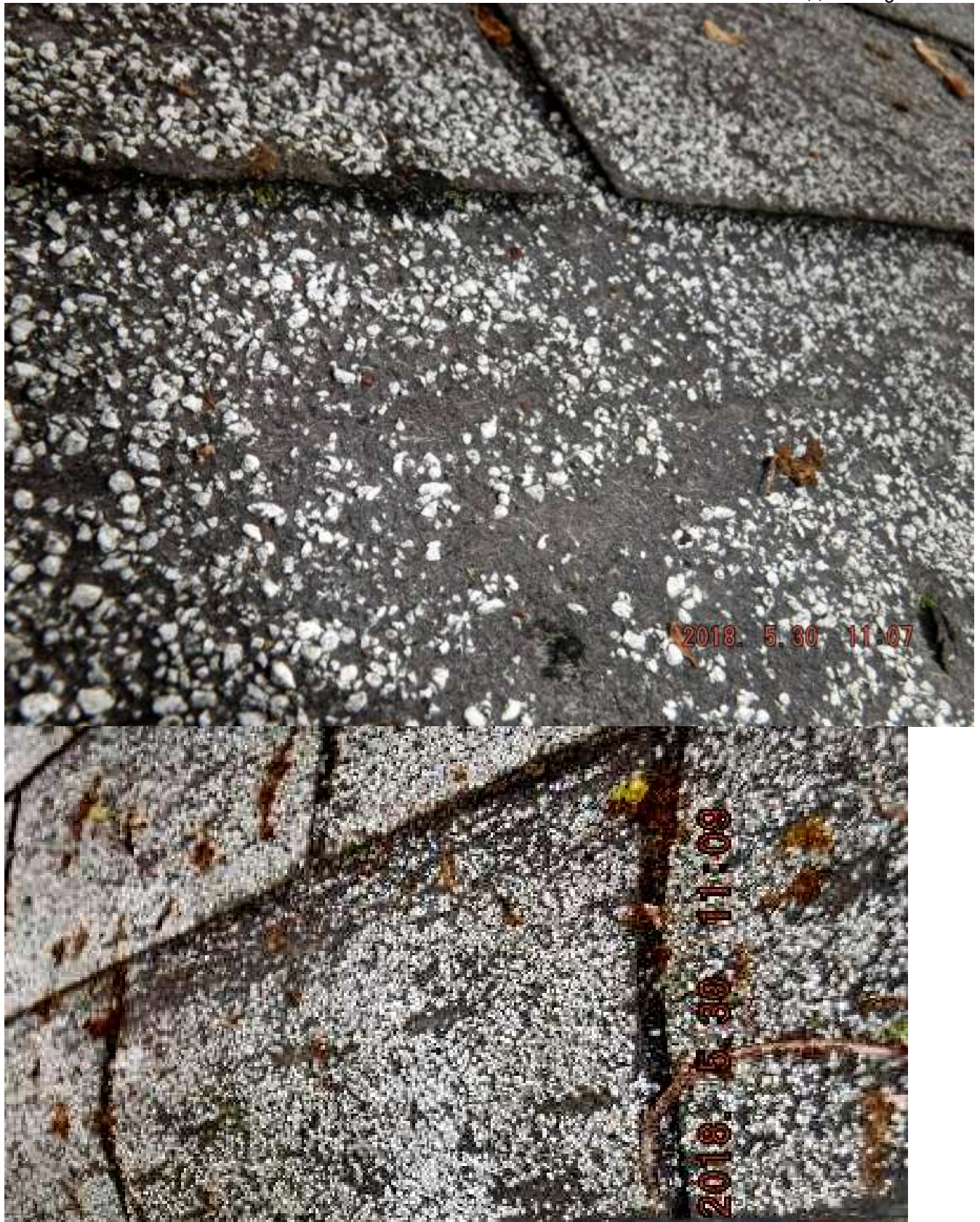
Figure 1 Example of extensive aggregate loss and exposed backing.
