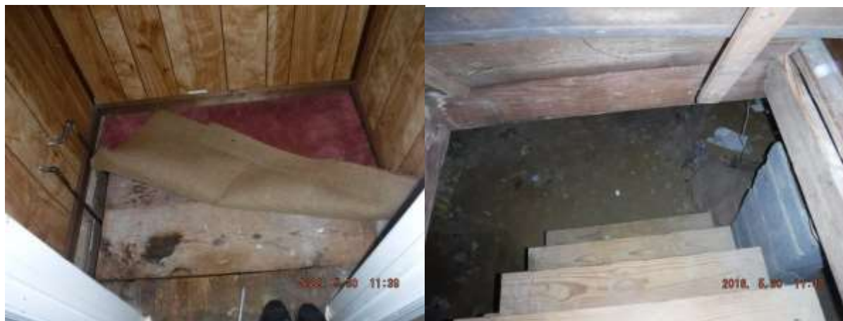
Figure 14 Recommend a carpenter evaluate floor hatch, steps and advise on upgrades, railing, etc. for safety.
