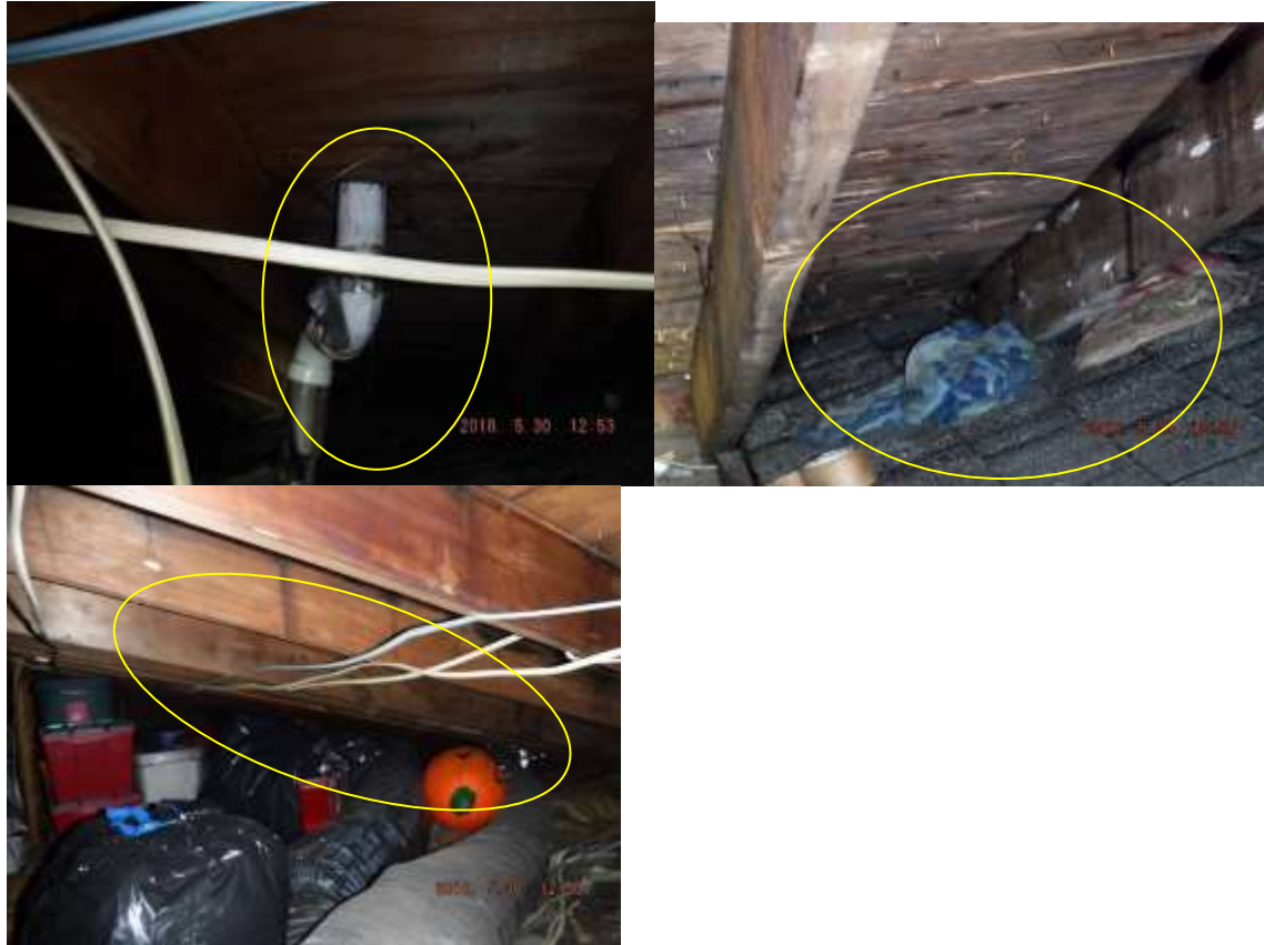
Figure 7 Example of packed storage in attic, wet rags under roof leaks, leaking roof penetrations, rusted nails, delamination/splits, etc.; poor roof condition.
