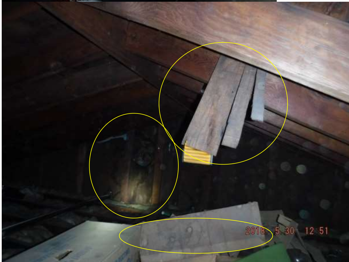
Figure 4 Example of water stains and peeled/delaminated sheathing (some hanging). Roof was poorly ventilated and leaking.
