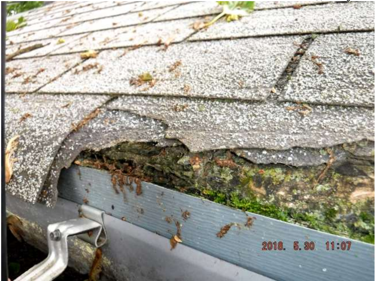
Figure 2 Example of damaged sheathing, moss, damaged shingles, etc.
