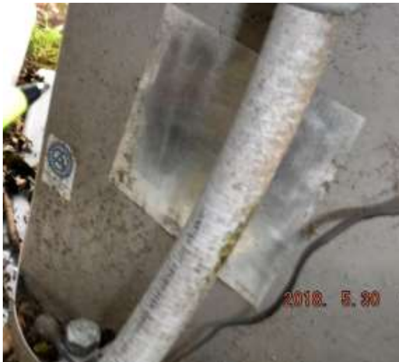
Figure 19 Data tag on condensing unit was worn off; appears very old.
