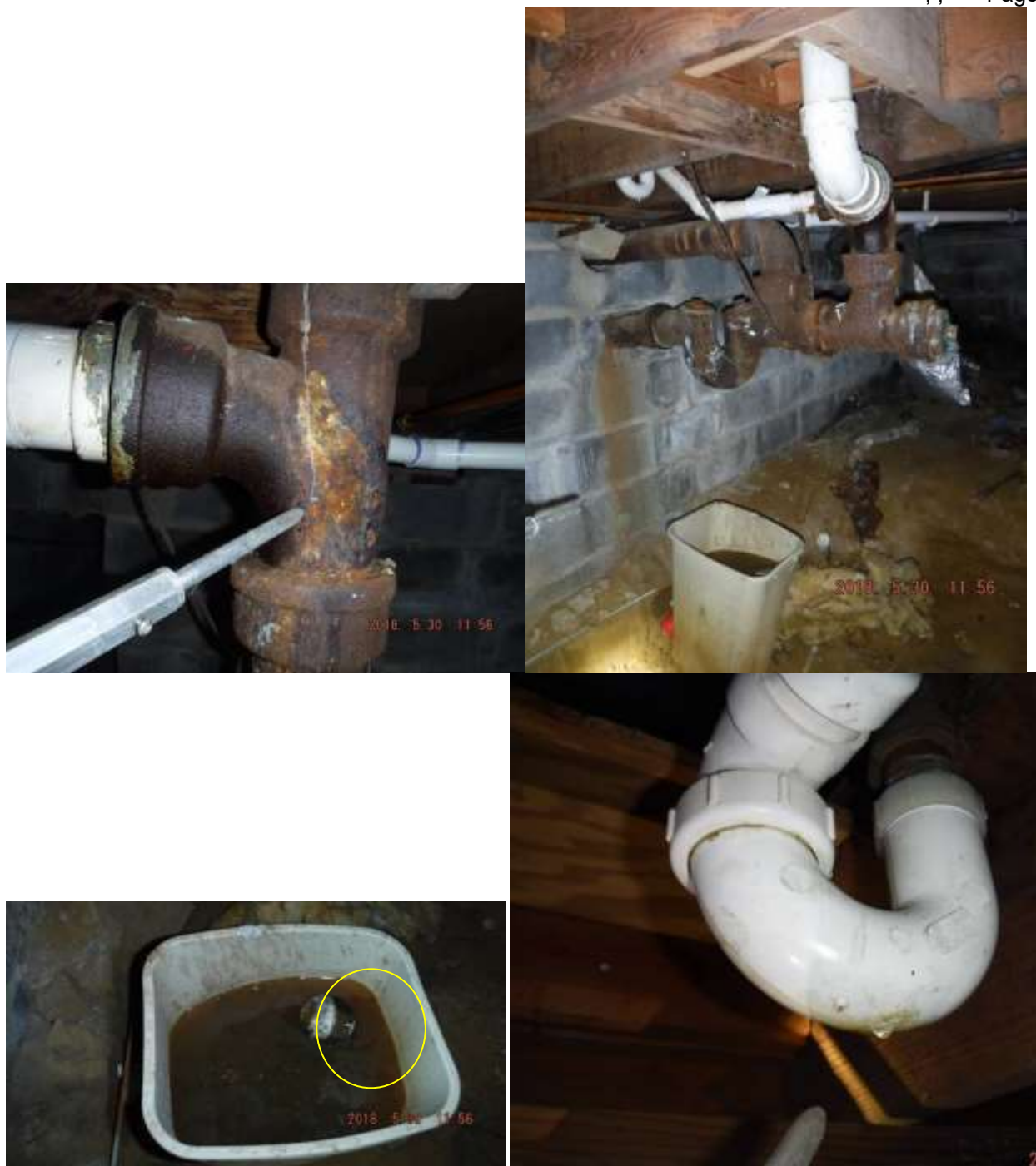
Figure 17 Example of corroded plumbing, leaking and brown water filled in a catch bucket. Recommend a licensed plumber evaluate all plumbing in home and advise on repairs/upgrades.
