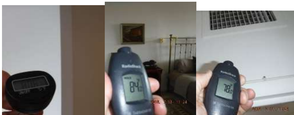
Figure 6 The A/C unit was on 70F when arrived and lowered and checked after an hour running at lower at lowest temperature to cool off home. The room temperatures were 78 at registers and 80°F in rooms and not cooling at all. The thermostat was not reflecting the 78-80F room temperatures and did not move from a 50F reading, which was incorrect.
