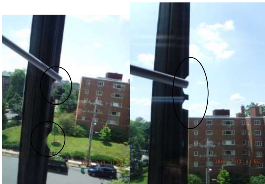
Figure 5 Windows in home were original ~ 43 yrs.; difficult to open/close, stiff, broken plastic frames, vapor seal breaks, etc.
