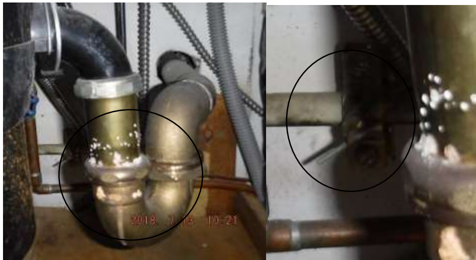
Figure 3 Example of corrosion on drain/plumbing under sink. There was a Tee saddle valve/piercing valve; tend to leak and considered handyman.
