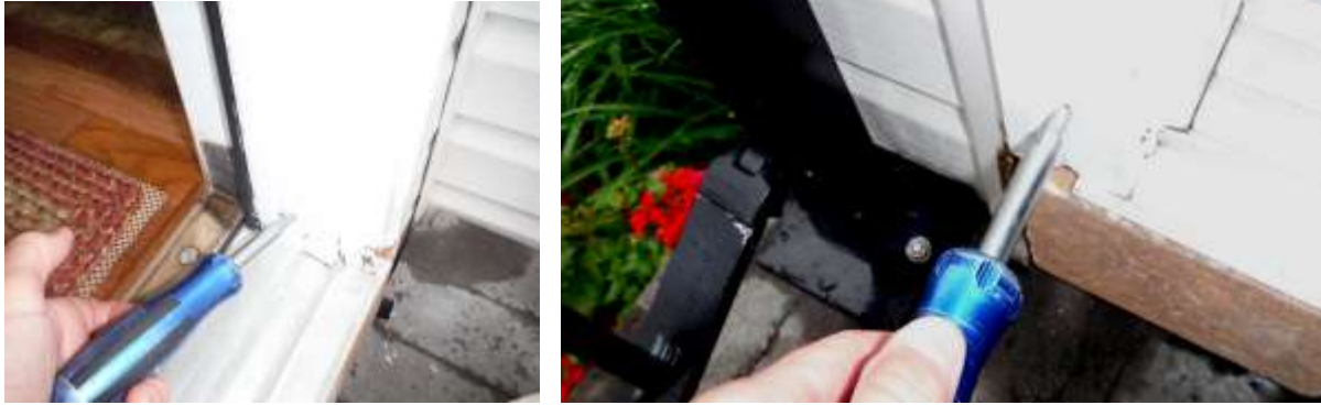
Figure 1 Have a structural carpenter evaluate extent of water/rot/damage on rear kitchen door and make repairs.
