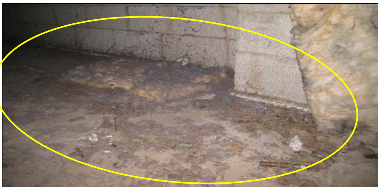
Figure 8 Heavy lint coating walls and floor in crawl space from disconnected dryer; correct venting and clean surfaces.
