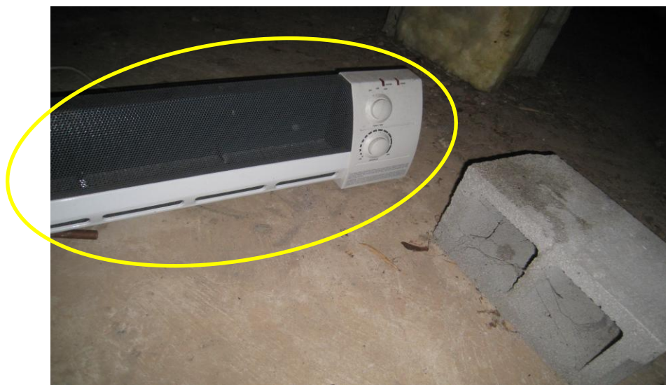
Figure 6 Long space heater under repaired pipes in crawl space; indication of freeze damage or improperly insulated plumbing.
