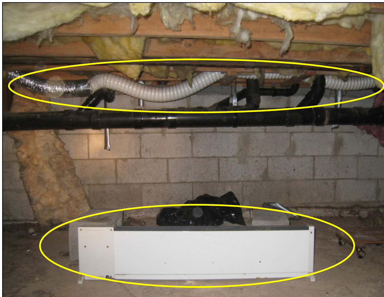
Figure 5 Electric Space heater below plumbing where repairs made. Have evaluated to install preventative measure to guard against freezing pipe, leaks, clogs and water main breaks. There is a flex vent disconnected on dryer and lint accumulating inside crawl space. Have ductwork replaced and clean yearly for fire safety.
