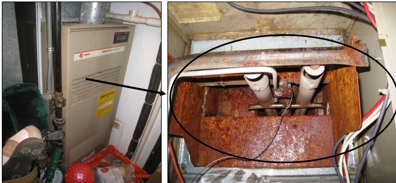
Figure 7 A & B Clutter poses a fire hazard in utility room. Heavy corrosion inside furnace; have evaluated now.
