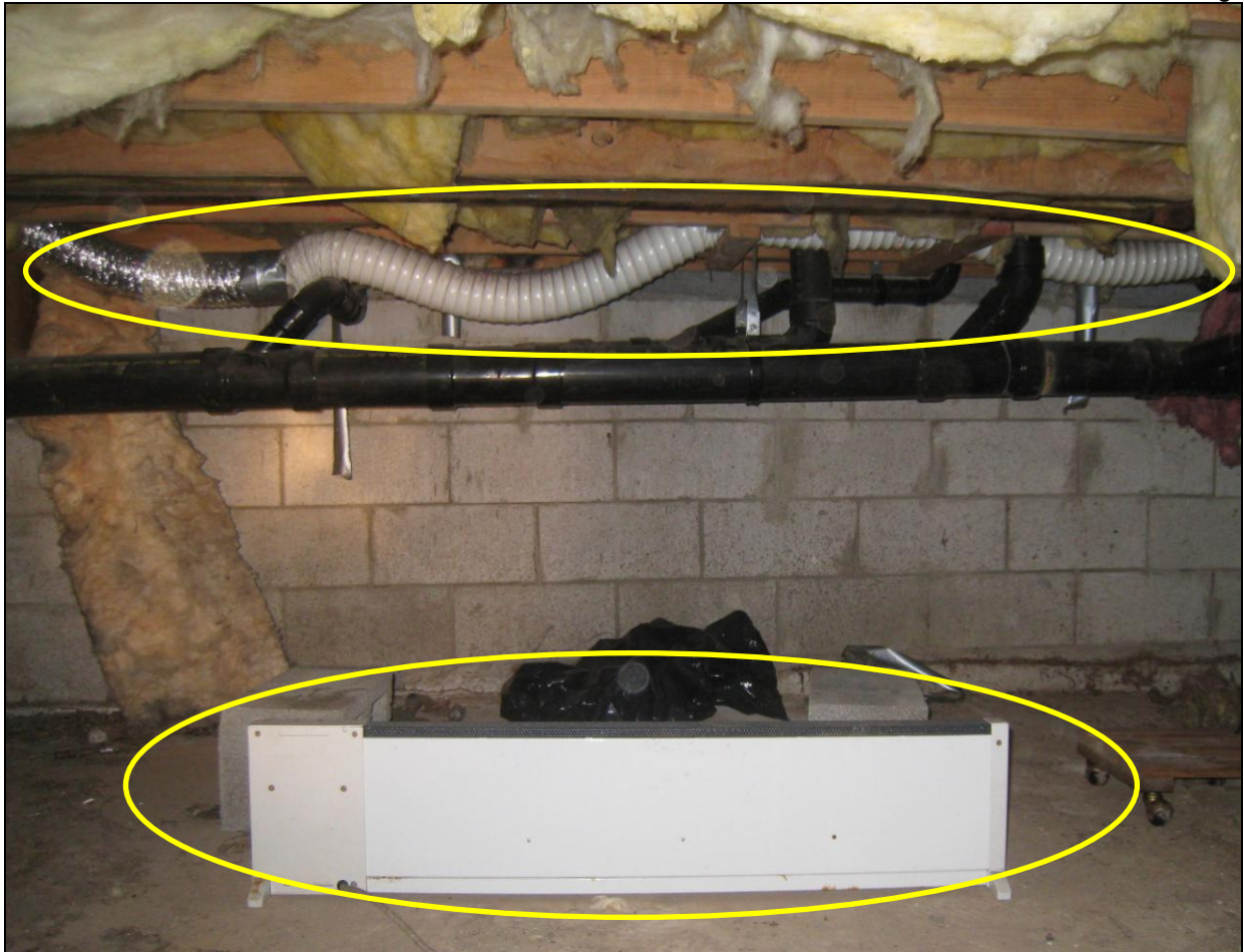
Figure 12 Electric Space heater below plumbing where repairs made. Have evaluated to install preventative measure to guard against freezing pipe, leaks, clogs and water main breaks. There is a flex vent disconnected on dryer and lint accumulating inside crawl space. Have ductwork replaced and clean yearly for fire safety.
