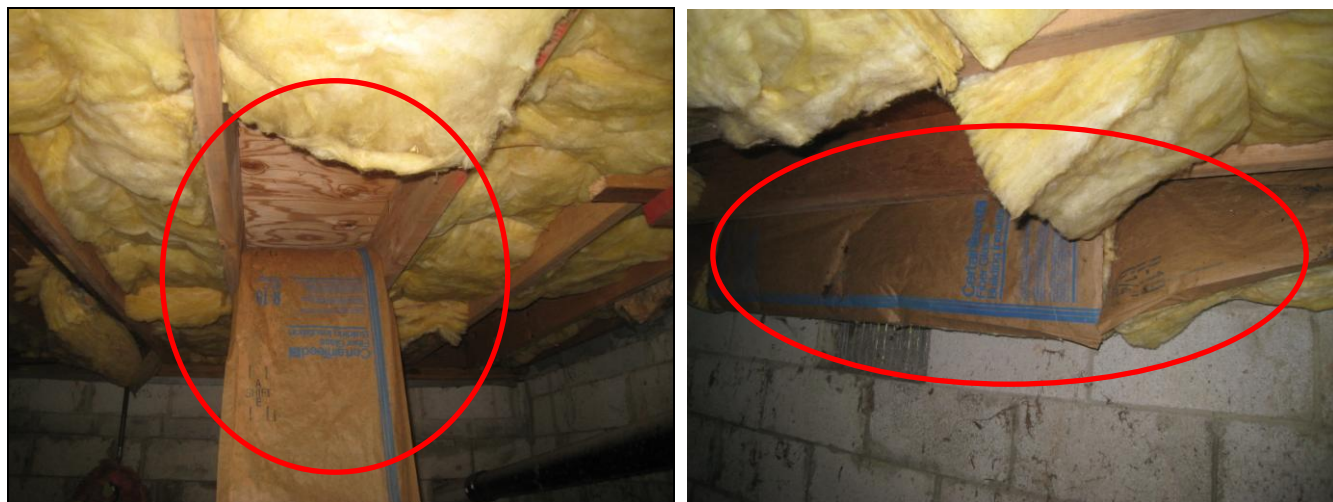
Figure 2 A & B Loose hanging insulation in crawl space.
