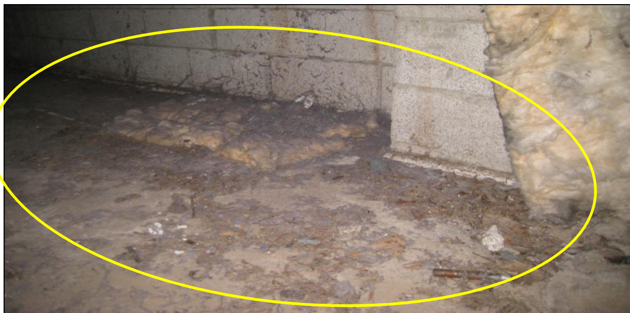
Figure 1 Heavy lint coating walls and floor in crawl space from disconnected dryer; correct venting and clean surfaces.
