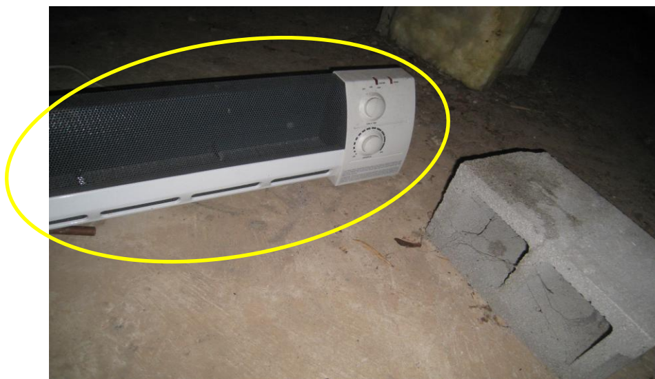
Figure 6 Long space heater under repaired pipes in crawl space; indication of freeze damage or improperly insulated plumbing.
