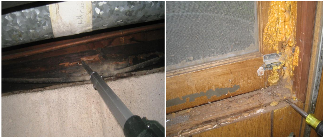
Figure 1 Sill damage, wood destroying insect. Have structural carpenter evaluate extent of all damage. Potential damage behind all wall and ceiling coverings.
