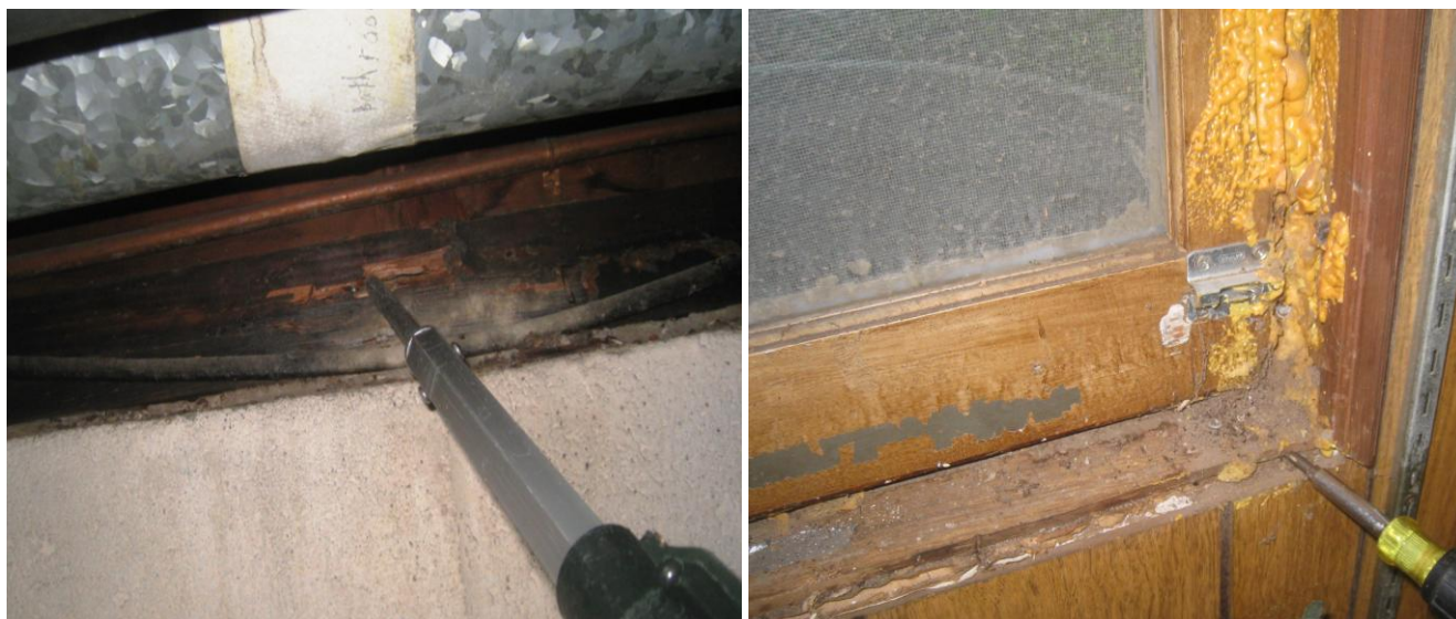
Figure 2 Sill damage, wood destroying insect. Have structural carpenter evaluate extent of all damage. Potential damage behind all wall and ceiling coverings.
